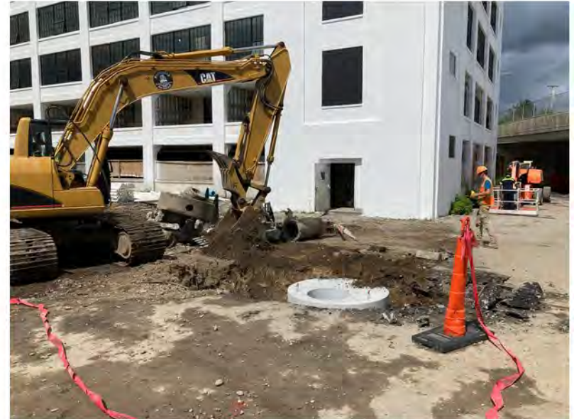
2022-08-23 13:46 42.1150639 N , 75.9505000 W Installation of sewer manhole structure at eastern end of Helen Drive
