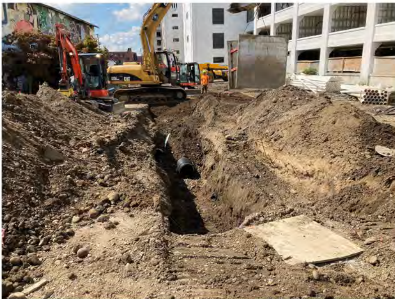
2022-08-24 14:49 42.1151194 N , 75.9505000 W Installation of storm sewer at eastern end of Helen Drive
