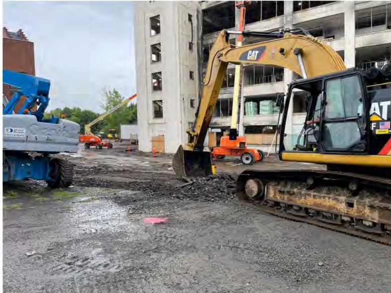
2022-08-22 08:42 42.1155028 N , 75.9526833 W Work Zone #1 (Southern Excavations) - Removal of asphalt in southwestern parking lot (northwestern portion)
