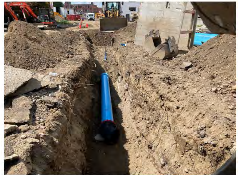
2022-08-25 13:47 42.1151194 N , 75.9504778 W Installation of water line at eastern end of Helen Drive
