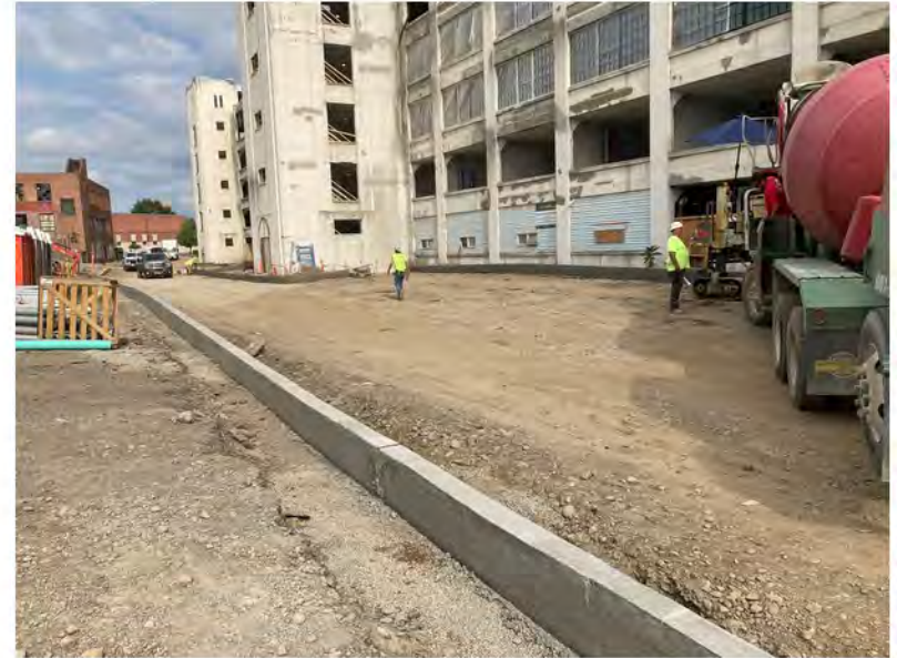
2022-08-30 10:01 42.1154222 N , 75.9518194 W Installation of curbs along Helen Drive, looking west from the intersection of Helen Drive and Avenue A
