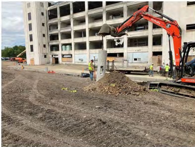
2022-08-30 13:20 42.1153028 N , 75.9523167 W Installation of light pole foundations in the parking lots along Helen Drive, looking northwest
