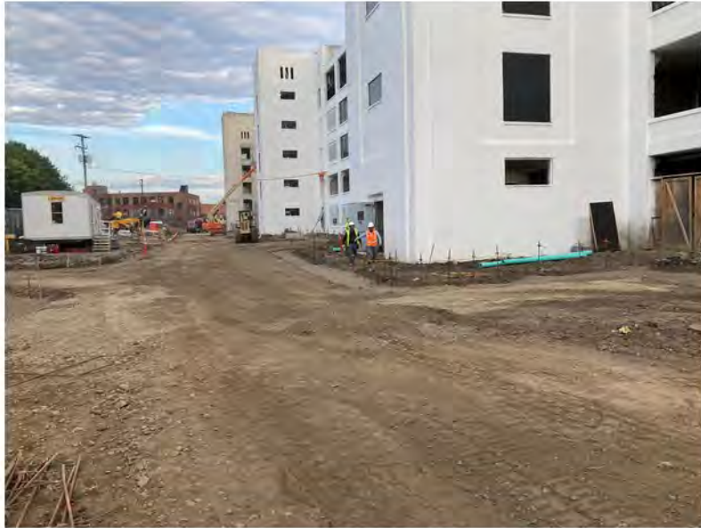
2022-08-30 07:32 42.1153833 N , 75.9508889 W Status of work along Helen Drive, looking west from the east end of the site
