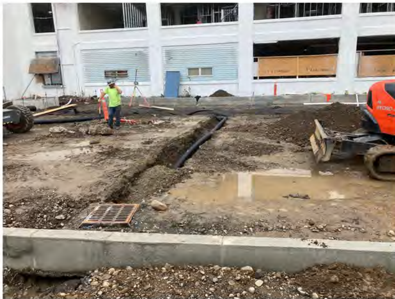
2022-09-07 13:10 42.1152611 N , 75.9515917 W Installation of drainage lines along Helen Drive between Avenues A and B, looking north
