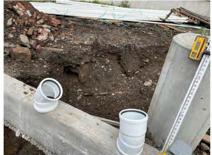
2022-09-08 11:52 42.1152694 N , 75.9507222 W Installation of water line near east end of building. Note that the structures/elbows are not part of the installation.
