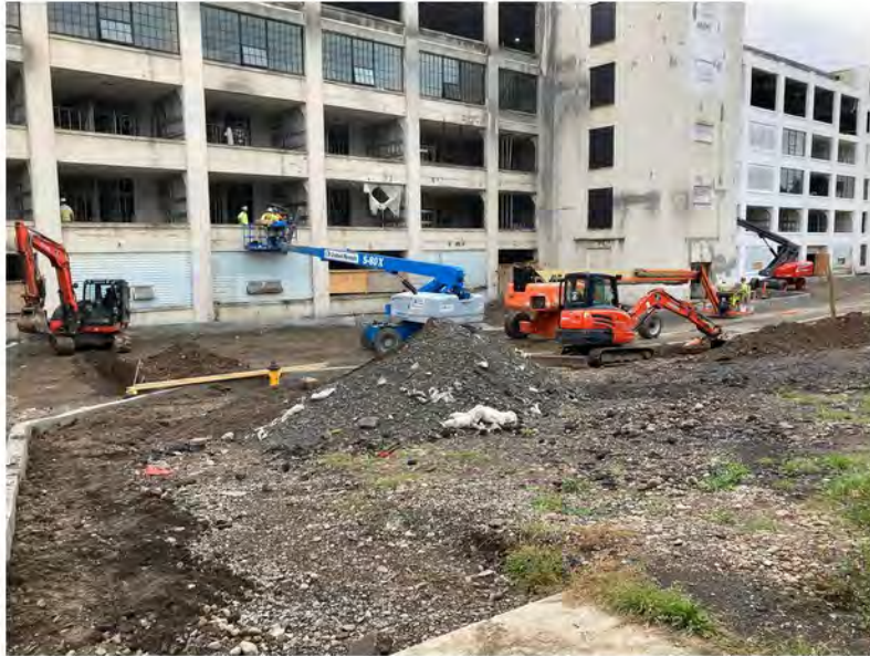
2022-09-06 09:27 42.1155611 N , 75.9529111 W Installation of electric conduit along Helen Drive near Avenue B, looking north
