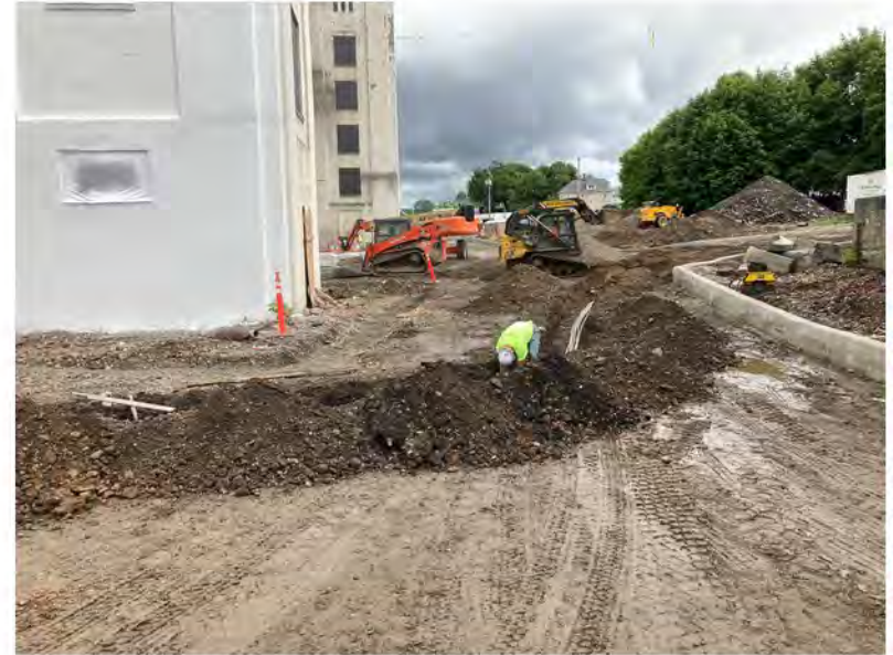
2022-09-06 14:16 42.1157806 N , 75.9532250 W Installation of electric conduit along Helen Drive near Avenue B, looking east
