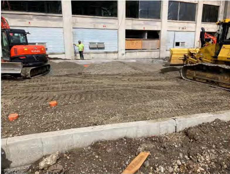
2022-09-13 14:08 42.1155056 N , 75.9527806 W Placement of road bedding along western portion of Helen Drive (on top of demarcation barrier).
