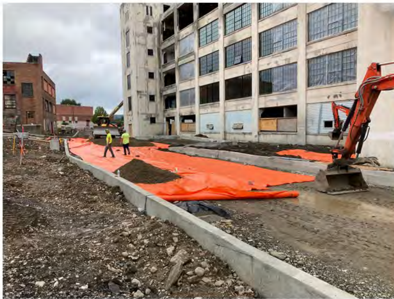
2022-09-13 12:50 42.1155139 N , 75.9523250 W Placement of demarcation barrier along western portion of Helen Drive.
