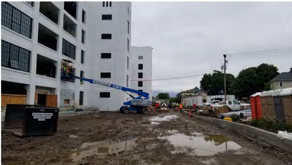
2022-09-13 09:25 42.1154627 N , 75.9522014 W Helen Drive near central portion of the site, looking east.
