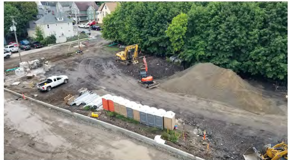
2022-09-13 09:42 42.1166012 N , 75.9527544 W Aerial view of eastern portion of southwestern parking lot, looking southeast.
