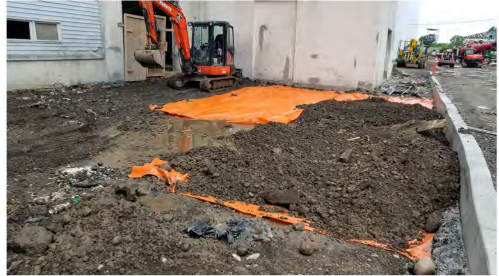
2022-09-13 11:51 42.1152294 N , 75.9521981 W Placement of demarcation barrier and cover material between the southern building facade and Helen Drive.
