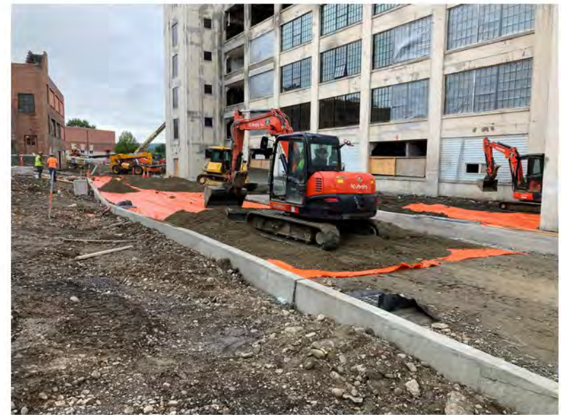
2022-09-13 12:58 42.1146861 N , 75.9528056 W Placement of demarcation barrier along western portion of Helen Drive.
