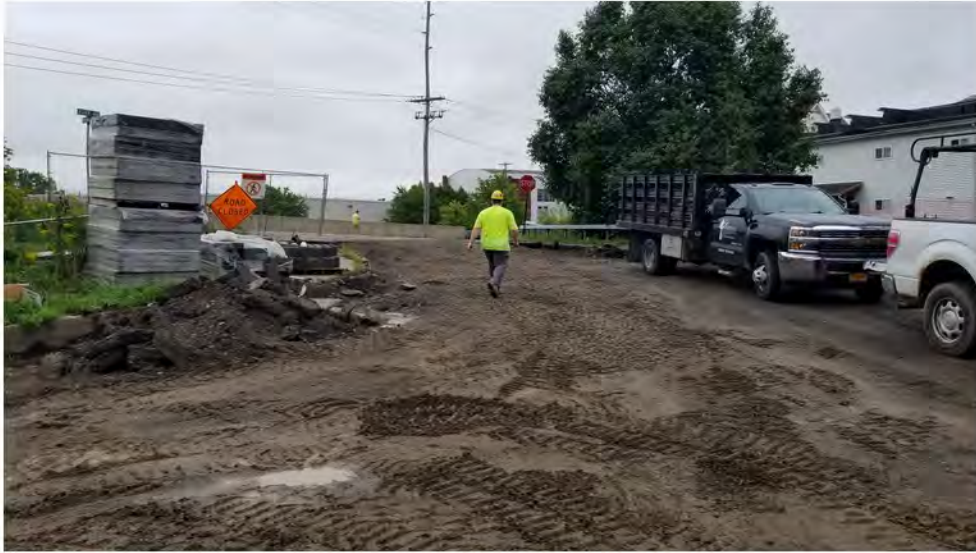
2022-09-13 09:28 42.1148085 N , 75.9508593 W Helen Drive at intersection with Lester Avenue, looking east.
