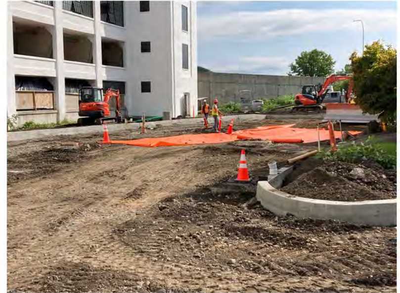
2022-09-14 11:39 42.1152528 N , 75.9511806 W Placement of demarcation barrier along eastern portion of Helen Drive.
