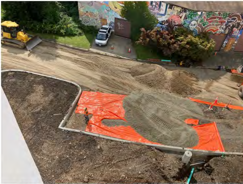
2022-09-14 13:15 42.1152528 N , 75.9509417 W Aerial view of placement of demarcation barrier along eastern portion of Helen Drive.
