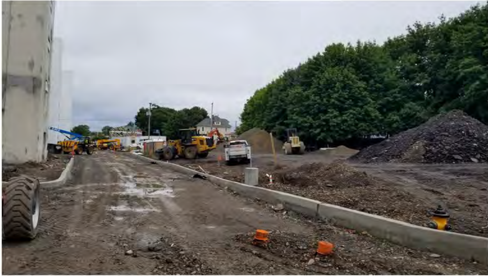
2022-09-13 09:19 42.1154079 N , 75.9522467 W Helen drive near intersection with Avenue B, looking east.
