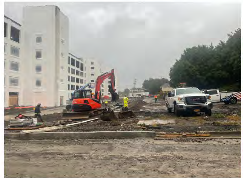
2022-09-22 07:59 42.1155778 N , 75.9529889 W Excavation associated with installation of electric conduit in southwestern parking lot, looking east
