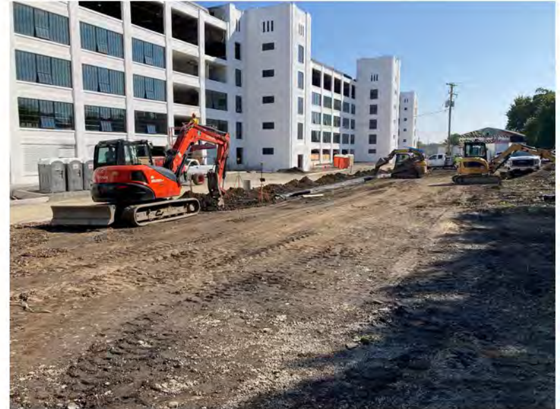
2022-09-21 11:06 42.1154556 N , 75.9525000 W Excavation associated with installation of drainage lines in southwestern parking lot, looking east
