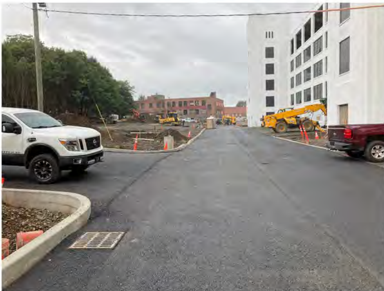
2022-09-28 10:20 42.1154833 N , 75.9514472 W Helen Drive (Work Zone #1) after paving, looking west. Demarcation barrier is located beneath pavement and gravel subbase in select areas (as detailed in RAWP).
