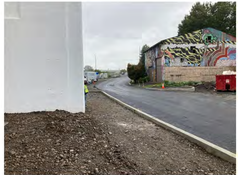
2022-09-28 10:20 42.1154222 N , 75.9512472 W Helen Drive (Work Zone #1) after paving, looking east. Demarcation barrier is located beneath pavement and gravel subbase in select areas (as detailed in RAWP).
