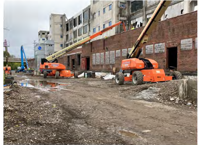
2022-09-26 11:51 42.1160278 N , 75.9522472 W Status of improvements in Work Zone #2 (Avenue C), looking east
