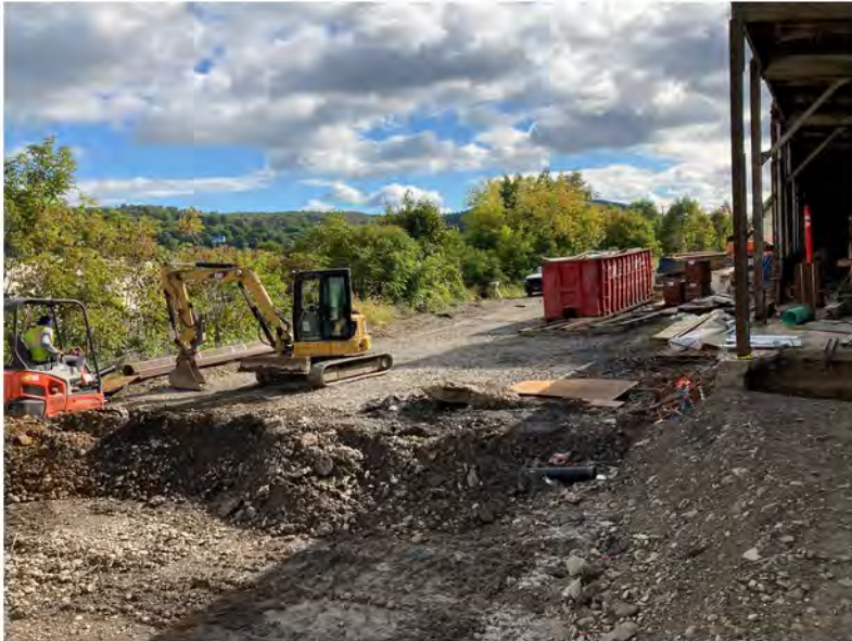
2022-09-26 10:06 42.1161028 N , 75.9528278 W Drain line installation in Work Zone #2 (Avenue C), looking east
