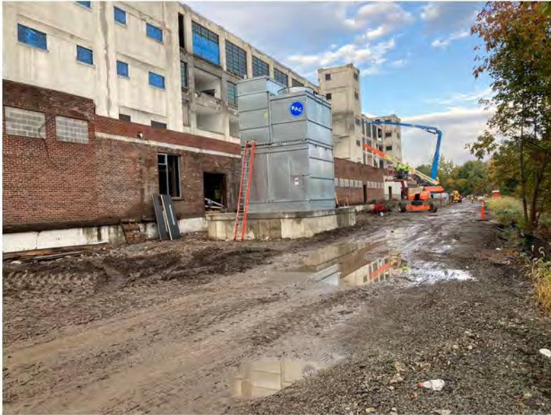
2022-10-07 08:34 42.1158361 N , 75.9513556 W Status of site work, northeastern section of Avenue C, looking west
