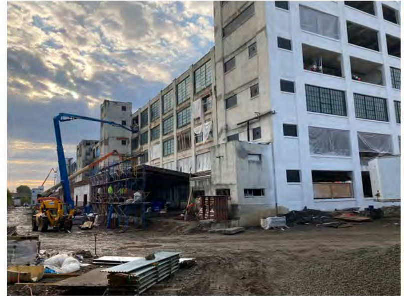
2022-10-07 08:36 42.1161611 N , 75.9530417 W Status of site work, northwestern section of Avenue C, looking east
