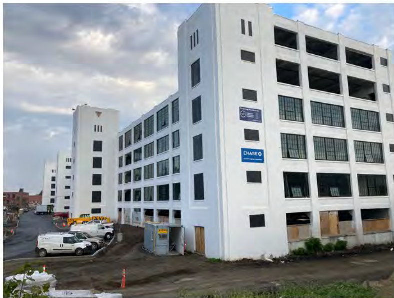
2022-10-07 08:24 42.1150889 N , 75.9503028 W Status of site work, eastern end of Helen Drive and Avenue C, looking west
