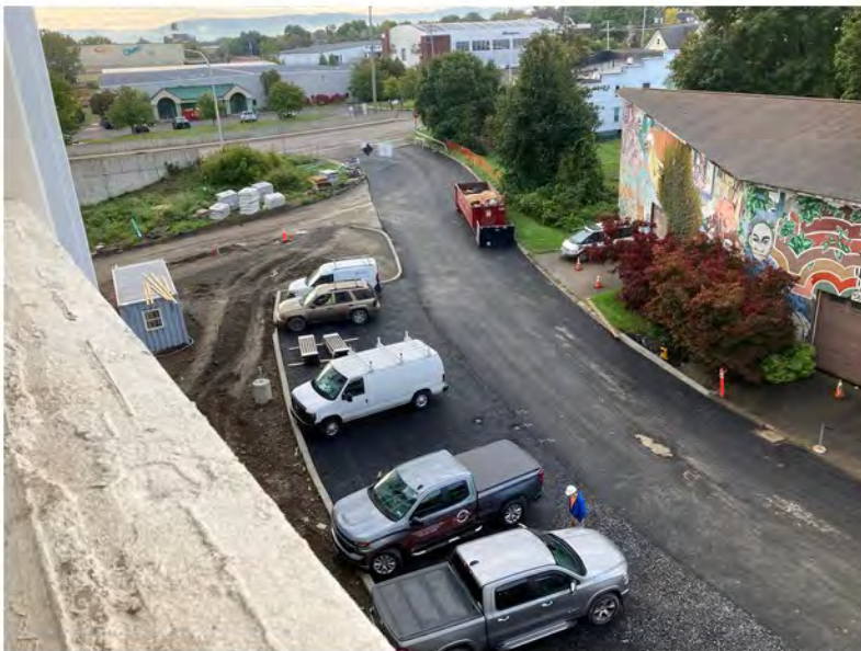
2022-10-07 08:58 42.1152611 N , 75.9509361 W Aerial view of eastern portion of Helen Drive, looking southeast
