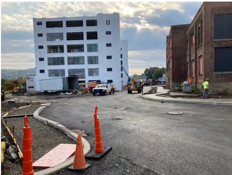
2022-10-07 08:38 42.1159056 N , 75.9536361 W Status of site work, western end of site, looking east
