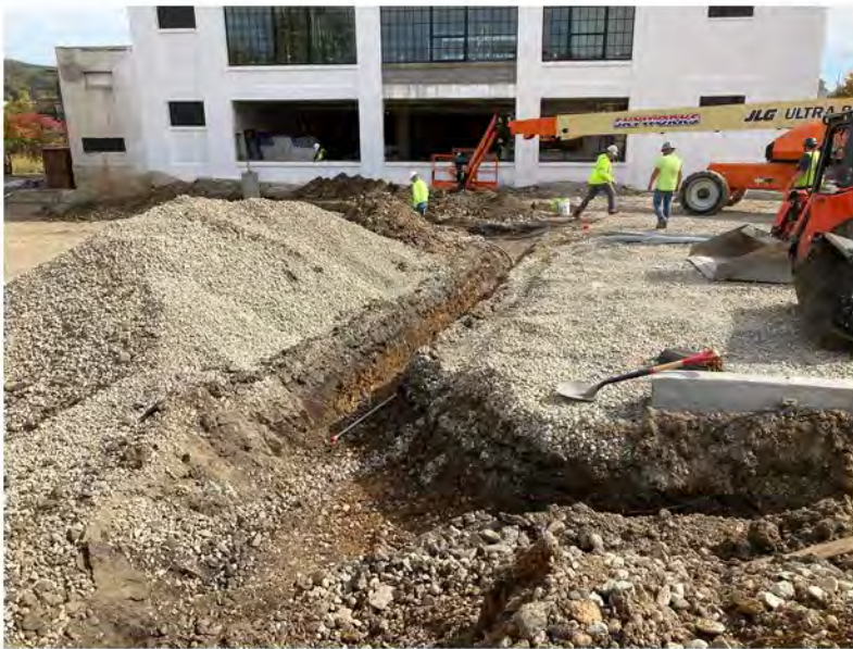
2022-10-12 12:54 42.1159750 N , 75.9531694 W Installation of electrical conduit at the western end of the site (Work Zone #1), looking east.
