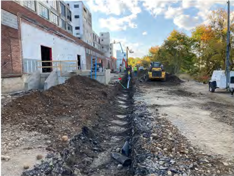
2022-10-11 15:59 42.1156417 N , 75.9508056 W Installation of water line along Avenue C (Work Zone #2), looking west.
