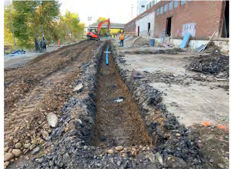
2022-10-11 16:11 42.1161639 N , 75.9515611 W Installation of water line along Avenue C (Work Zone #2), looking east.
