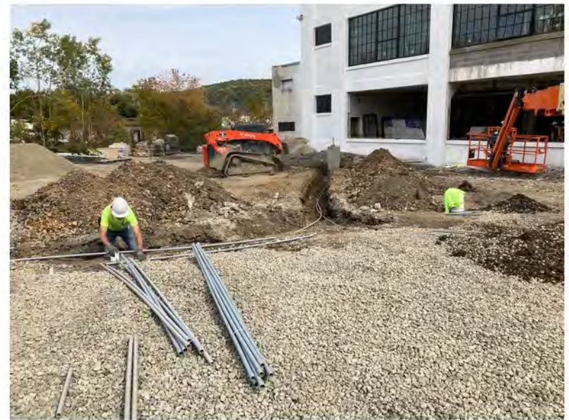
2022-10-12 13:22 42.1154139 N , 75.9525306 W Installation of electrical conduit at the western end of the site (Work Zone #1), looking north.
