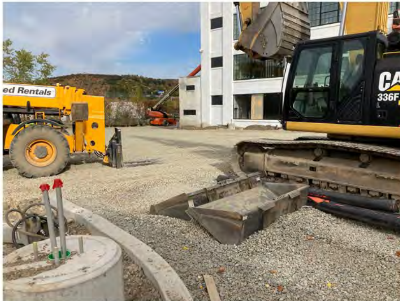
2022-10-20 15:28 42.1158778 N , 75.9532250 W Status of site work at the western end of the Site, looking northeast.
