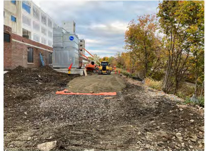
2022-10-19 07:53 42.1159389 N , 75.9511861 W Installation of demarcation barrier and roadway subbase along Avenue C, looking west.
