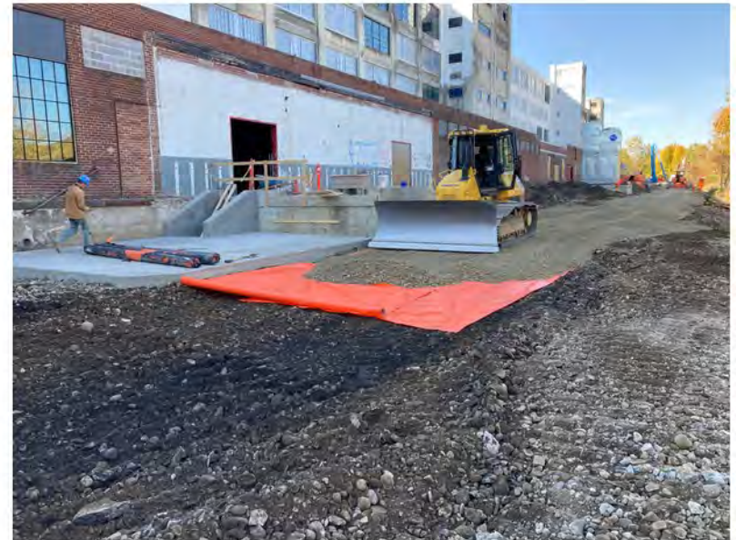
2022-10-21 12:31 42.1156833 N , 75.9507000 W Installation of demarcation barrier and roadway subbase along Avenue C, looking west.
