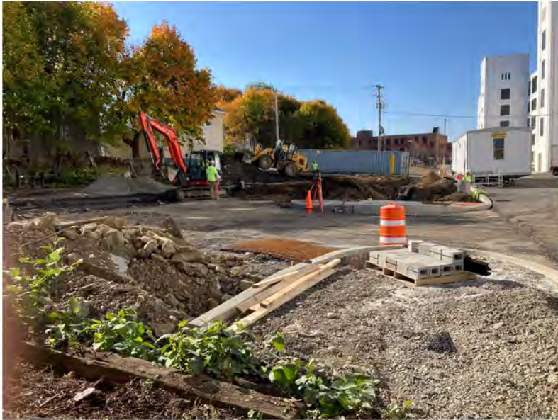
2022-10-21 15:03 42.1153500 N , 75.9509889 W Status of site work at the intersection of Avenue A (center) and Helen Drive (right), looking west.
