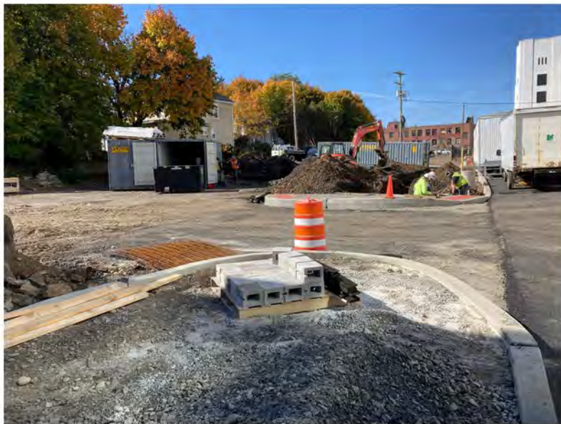
2022-10-21 12:33 42.1151667 N , 75.9511028 W Site work, including the installation of light poles and parking lot subbase, at the intersection of Avenue A (center) and Helen Drive (right), looking west.
