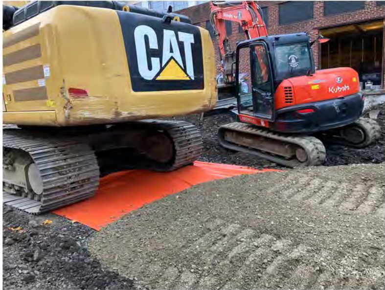
2022-10-19 07:27 42.1158444 N , 75.9514528 W Installation of demarcation barrier and roadway subbase along Avenue C.
