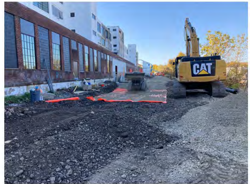
2022-10-21 14:38 42.1172639 N , 75.9480583 W Installation of demarcation barrier and roadway subbase along Avenue C, looking west.
