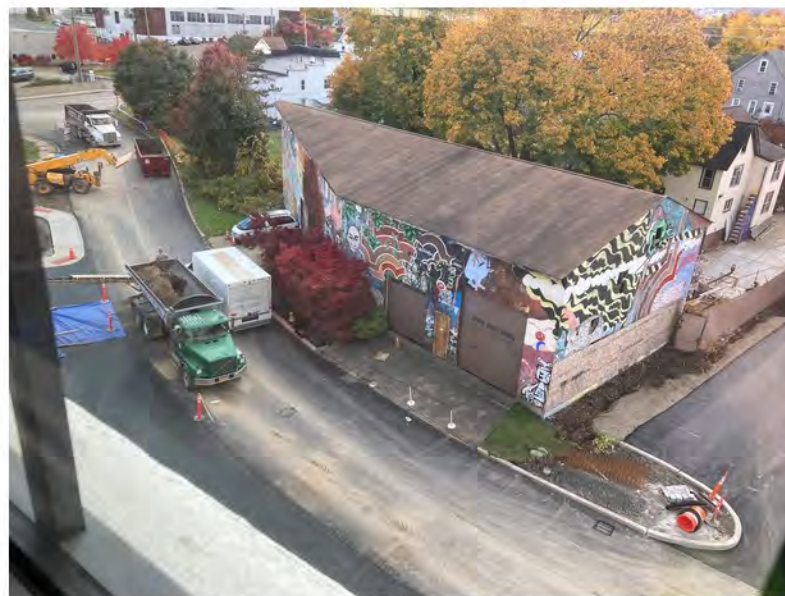
2022-10-25 13:09 42.1153750 N , 75.9510194 W Aerial view of eastern portion of Helen Drive, looking east
