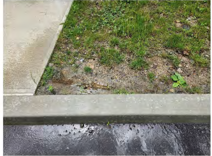
Area of thin lawn area on steep grade, immediately after a downpour. No erosion observed.
