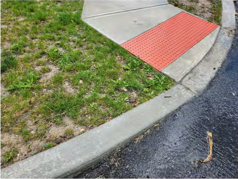
Area of thin lawn area on steep grade, immediately after a downpour. No erosion observed.
