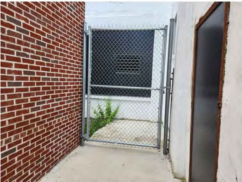
No tenant access to "courtyard" between main building and annex
