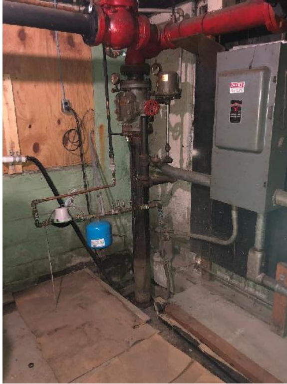
View of the basement sump pump and wooden curbing.
