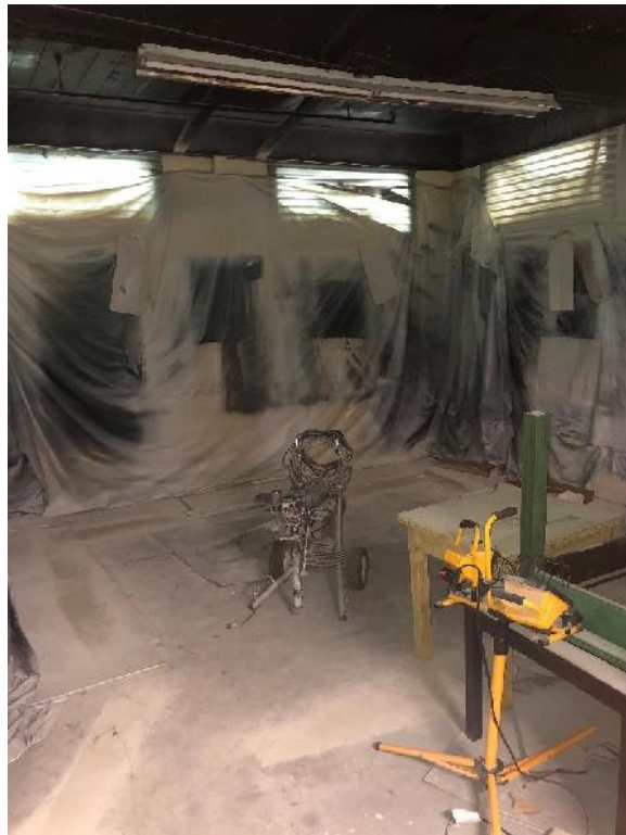
View of spray-painting booth in the northwest corner of the first floor.
