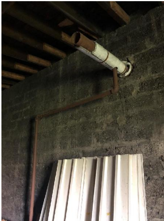
View of a pipe entering the former boiler room on the north of the building.
