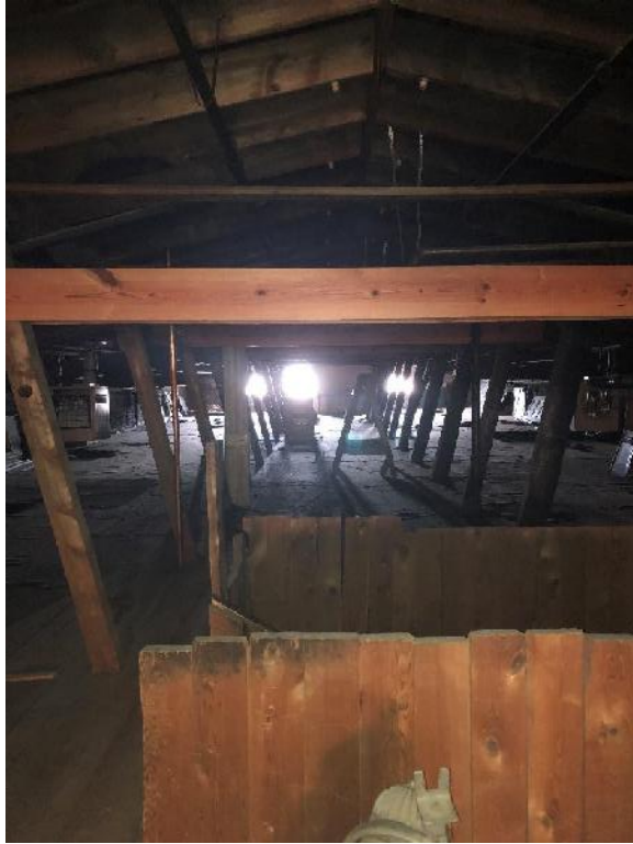
View of Subject Property Building third floor (attic) from the center staircase.
