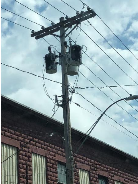
View of three electrical transformers located along Stockton Place.
