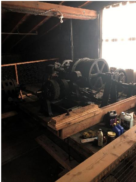
View of the mechanical elevator engine in the attic.
