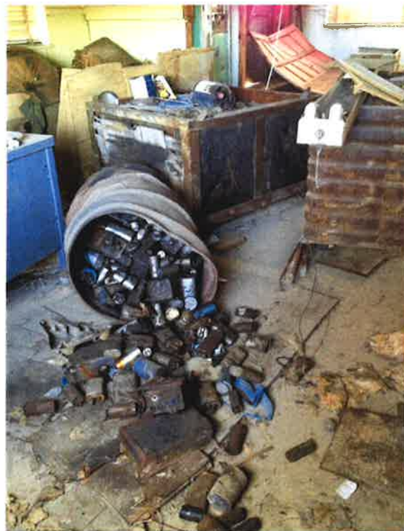
Photo 4 – Building 4 – potential PCB containing capacitors within building 4
