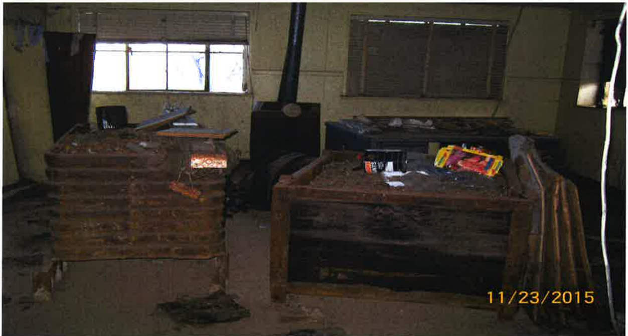
Photo 6 – Building 4 – Potential asbestos containing materials within building 4
