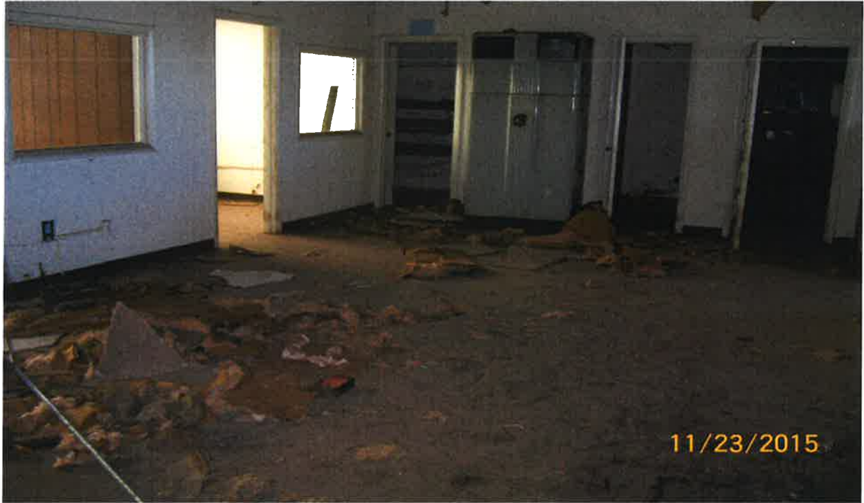
Photo 5 – Building 4 – Potential asbestos containing materials within building 4
