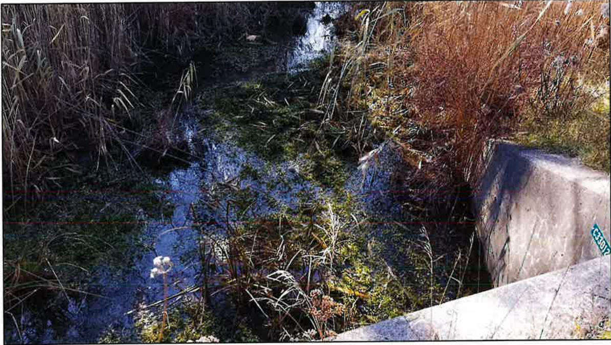
Photo: 41. Facing W at the intersection of the swale and culvert crossing of Interstate 690 (photo taken 11/15/2017).
