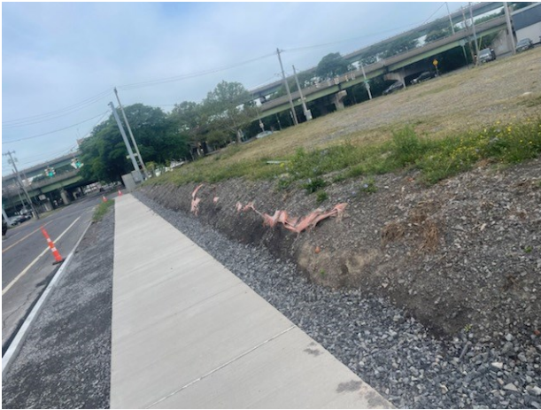
Photo of damaged to site cover and demarcation layer.
