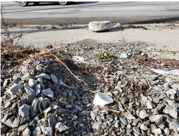
Photo of damage to monitoring well MW-4's protective casing/lid and PVC.
