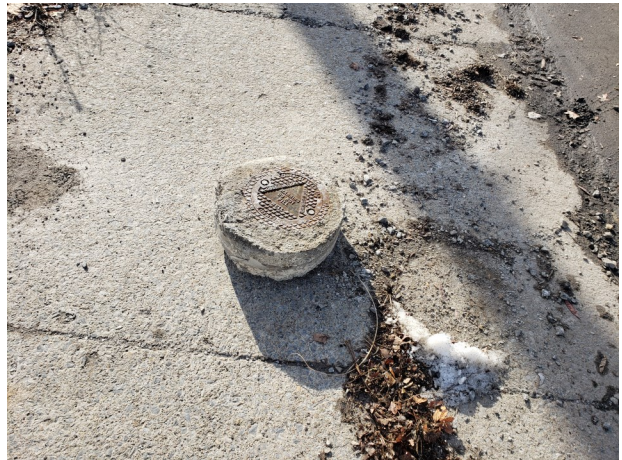
Photo of damage to monitoring well MW-4's protective casing/lid.
