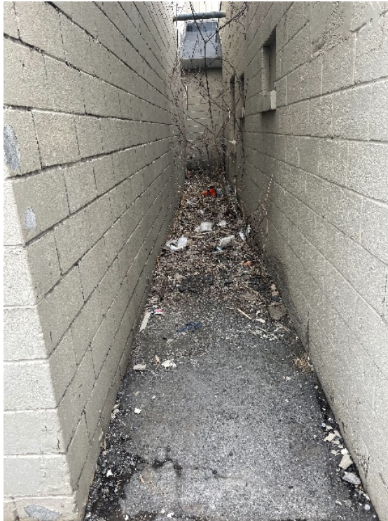
Photo 16 - View of trees in alleyway between building sections along Luther Avenue. Recommend trees be removed for integrity of soil cover engineering control.
