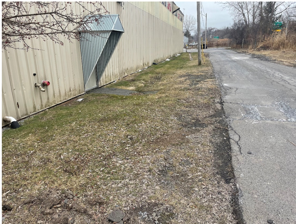
Photo 2 - View of minor soil rutting along Albion Avenue (not on the BCP Site). Recommended to be repaired when weather conditions allow.
