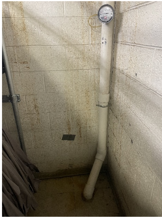
Photo 13 - View of typical SSDS suction point riser and magnehelic gauge.
