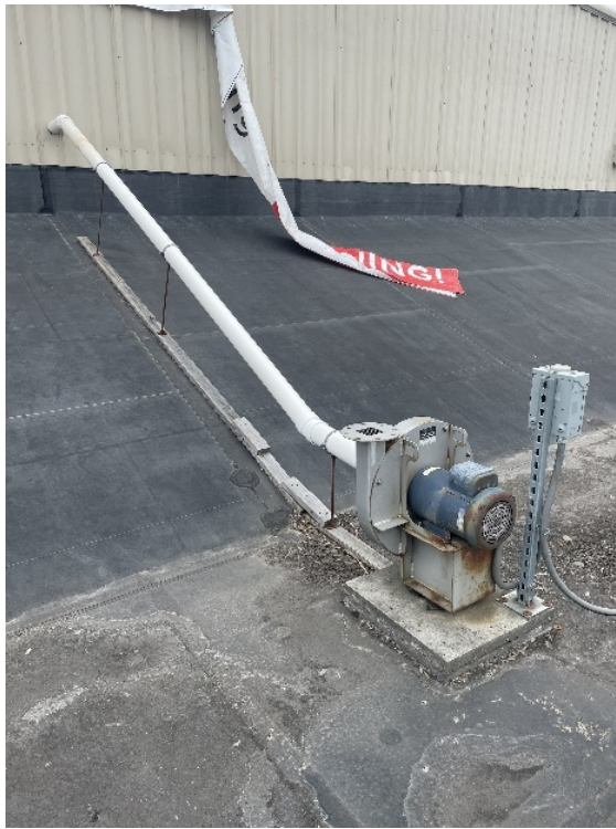
Photo 9 - View of Fan 1 and pipe supports. Recommended repairs were made by Box Capital in April 2020.
