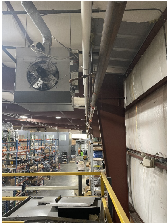
Photo 12 - View of SSDS main trunk line piping through main warehouse portion of Site building.
