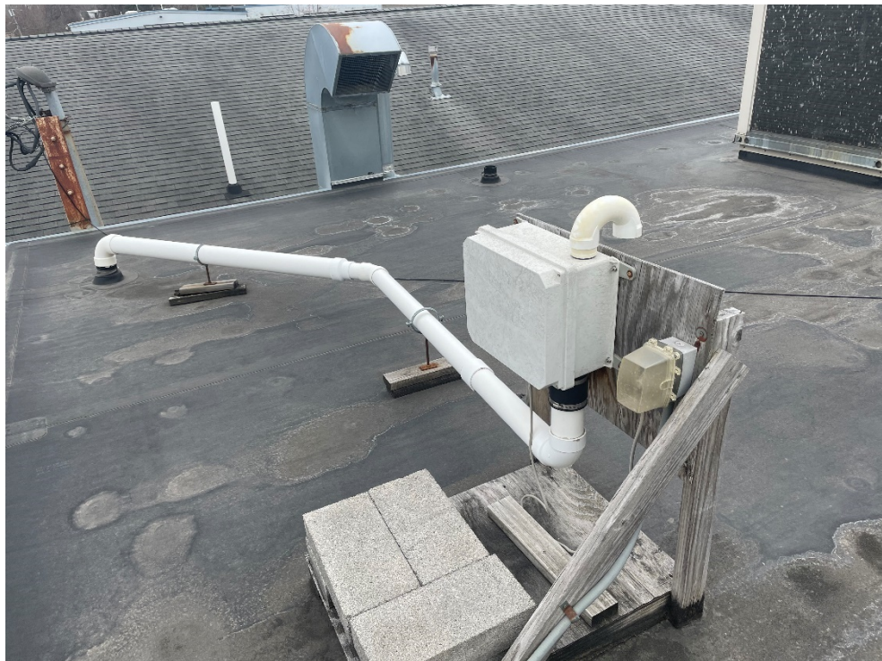
Photo 14 - Photo of SSDS Fan 2 on southern roof of building near Luther Avenue.
