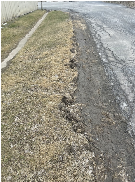
Photo 1 - View of minor soil rutting near western corner of building along Albion Avenue (not on the BCP Site). Recommended to be repaired when weather conditions allow.
