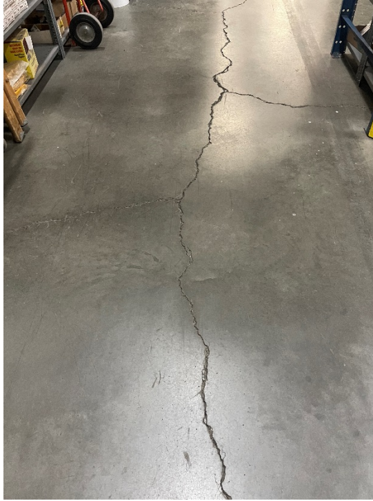
Photo 17 - View of surface cracks in interior concrete floor slab located in main warehouse portion of building. Recommended to be repaired or sealed for integrity of soil cover engineering control and/or to prevent potential short-circuiting of the SSDS in this portion of the building.
