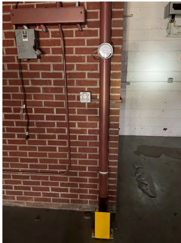
Photo 9 Typical view of riser piping with bollard and magnehelic gauge.
