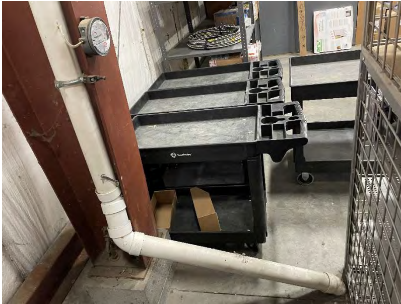
Photo 3 Typical view of riser with magnehelic gauge in warehouse area.
