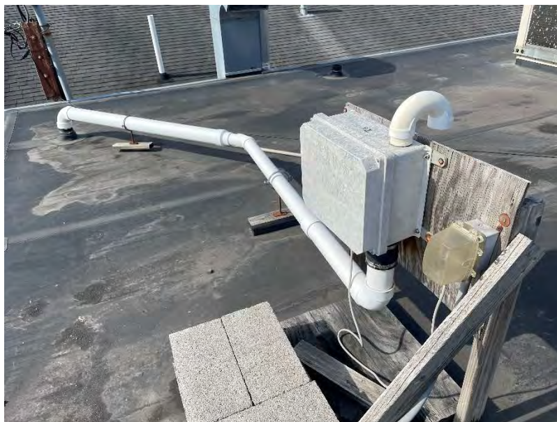
Photo 6 Typical view of header pipe and exhaust fan located on the roof.
