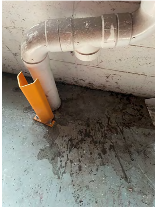
Photo 7 View of riser piping showing bollard and potential leak at knockout from condensation or water intrusion into exhaust fan.
