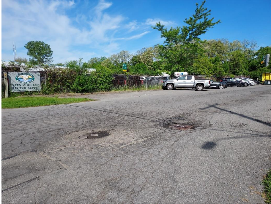
Photo 9 View of asphalt pavement deterioration along western side of Site.
