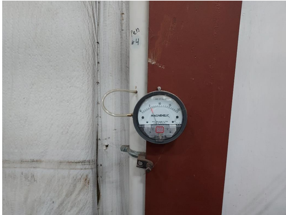
Photo 1 View of typical SSDS suction riser magnehelic gauge.
