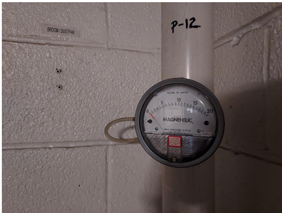
Photo 4 View of typical SSDS magnehelic gauge in southern portion of building, used for warehouse space, showing low reading because roof-mounted blower was non-operational.
