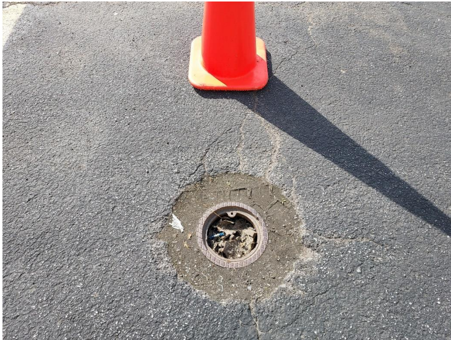
Photo 16 View of groundwater monitoring well MW-8 that was found to be missing its cover. The cover was replaced following the May 2025 groundwater monitoring event.
