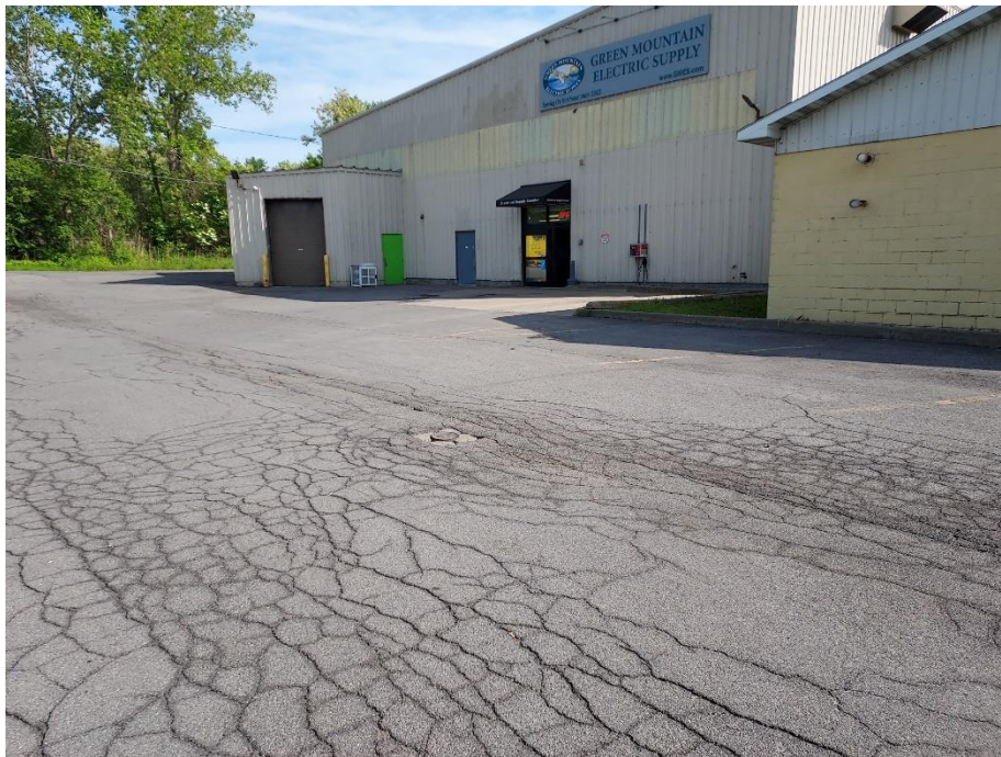
Photo 10 Another view of asphalt pavement deterioration along western side of Site.
