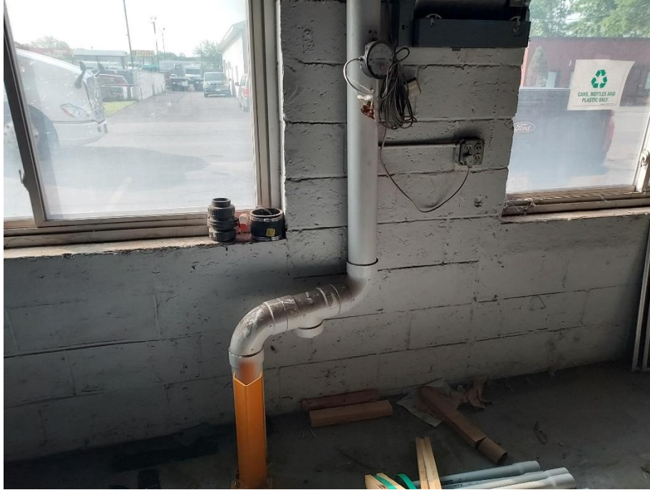
Photo 3 View of typical SSDS suction riser with bollard protection.
