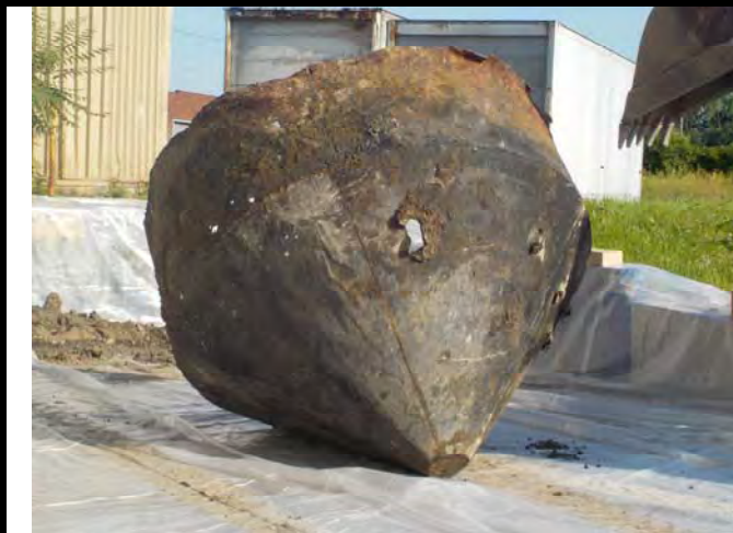
Photograph 25. First tank removed. Holes and thin steel noted at the bottom of the tank.
