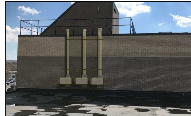
Figure 3.01Cii: Sketch of sidewall mounted fans on existing photo at roof elevation change.
