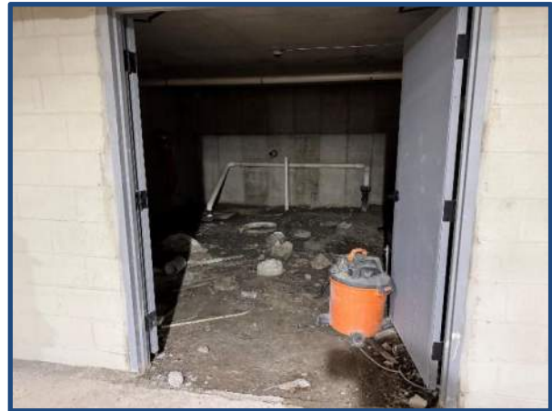
Basement Level, Southwest Utility Room, with Exposed Soil
