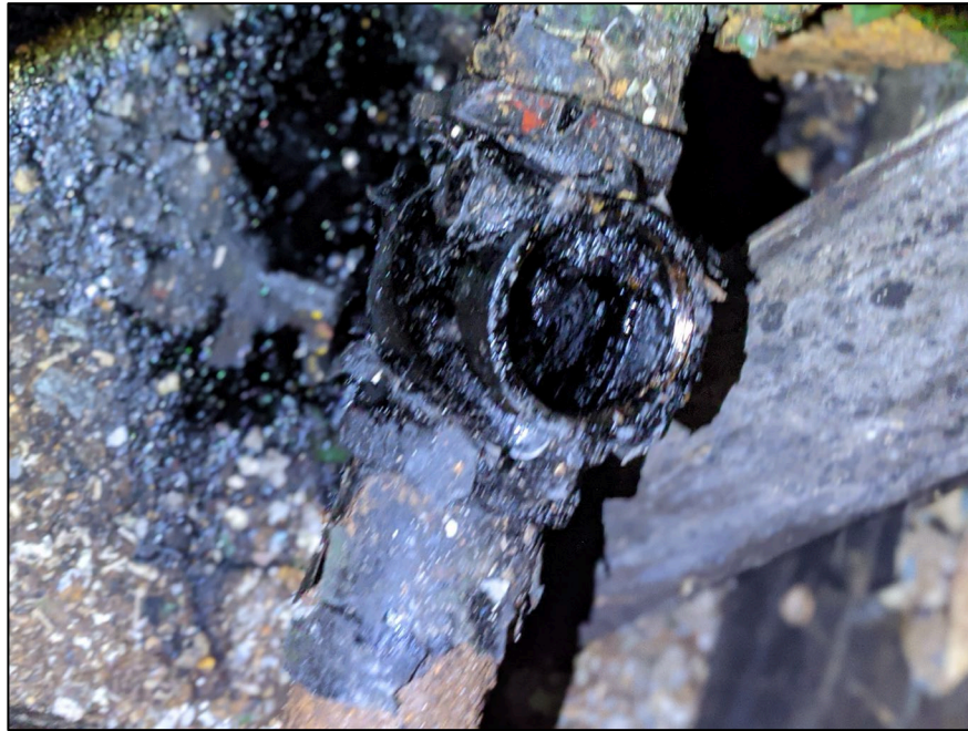
Exhibit 1-3 Accumulated Oil in Open Pipeline in Boiler Room
