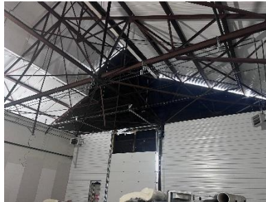
View of Gaps at Exterior Siding in the Barn
