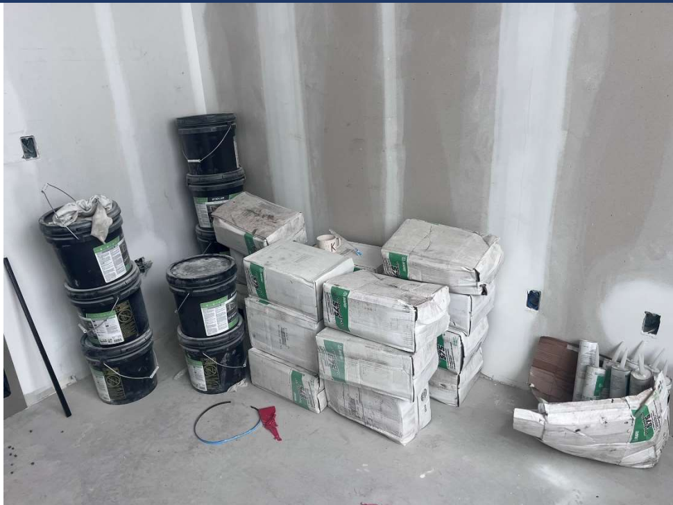
View of UltraBond Eco 575 and Taylor Signature Line Dynamic Adhesive stored in the Main Building.
