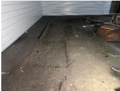
View of Minor Floor Cracking in the Barn
