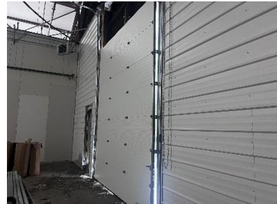
View of Gaps at Garage Door in the Barn
