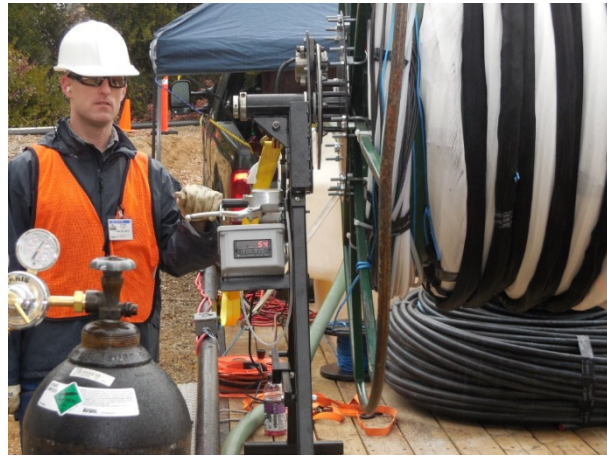
Fig. 7.1.4. FLUTE braking system for lowering Water FLUTE PVDF pumping system into borehole with deep water table.
