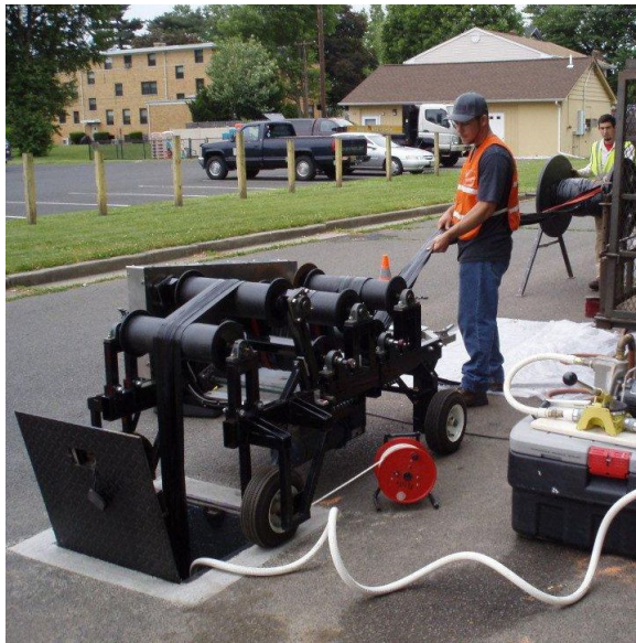
Fig. 3.2.2. The FLUTE Linear Capstan showing the zigzag path of the liner through the chain driven rollers with a variable speed motor drive and tension measurement. With minimum hand tension, the machine can pull more than 500 lb. of tension on a liner.
