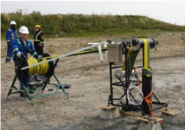
Fig. 5.2.2. Photo of profiling equipment in the field. The data is recorded to a laptop computer during the installation. Water is usually pumped from a tank into the liner to maintain a nearly constant driving pressure in the borehole.
