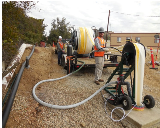
Fig. 7.1.3. Water FLUTE being installed in a 600 ft., 6 inch diam. borehole with 12 ports. The Green Machine is being used as wellhead roller to align liner with borehole. The grey hose and valve are for water addition to liner.
