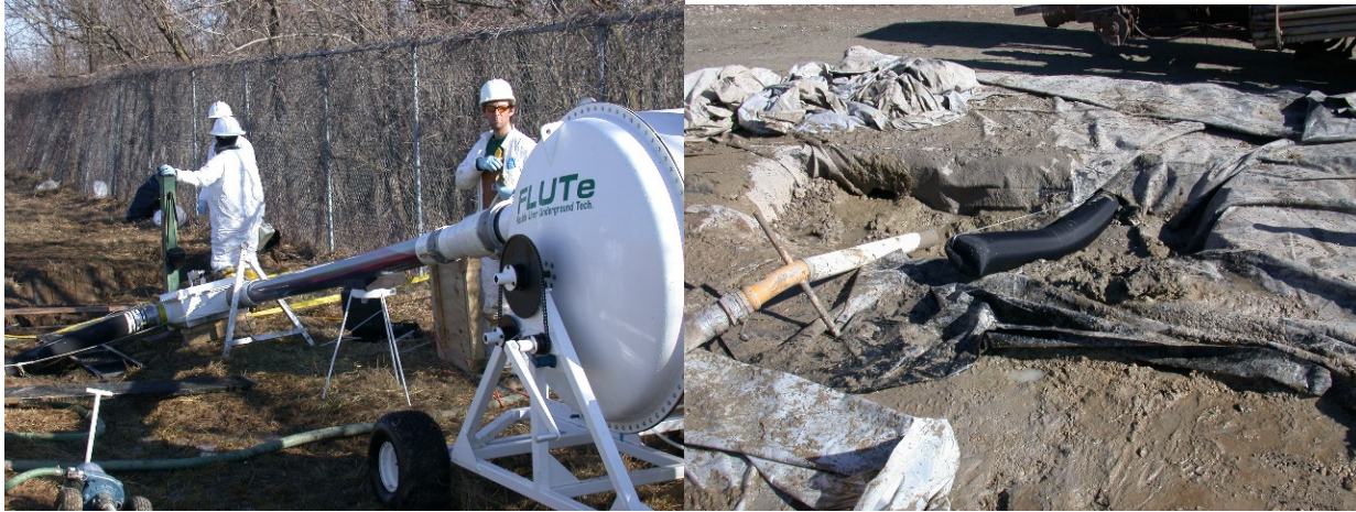
Fig. 9.1.3 LAHD installation from canister following the reamer under a landfill. Liner is shown everting out of horizontal hole 400 ft from the entrance. Liner is still clean because it was everting through the mud. The liner emplaced 8 sampling ports under the landfill.
