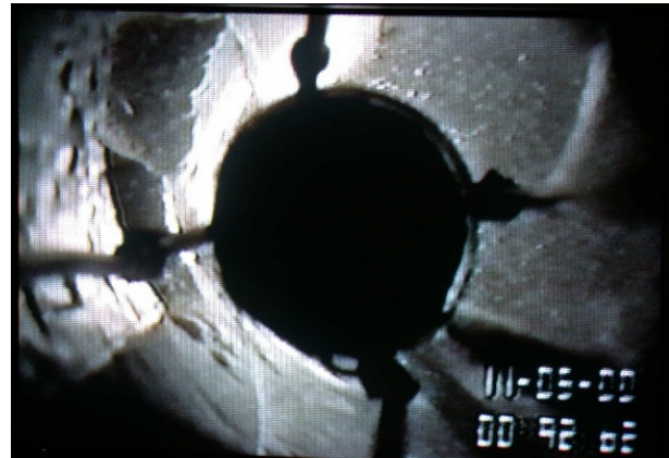
Fig. 3.2.4. Snapshot of the interior of a liner showing how well the liner conforms to the vugs in the borehole wall and the ledge in upper left of photo. (Large black central object is the back of the light source.)
