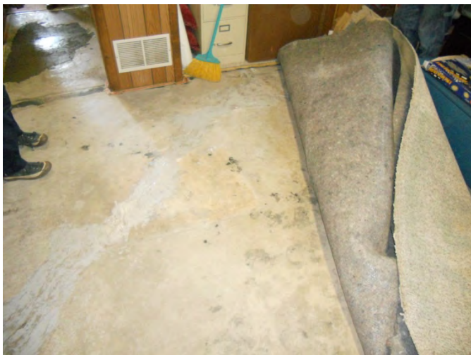
Sealed floor cracks –Structure 35
