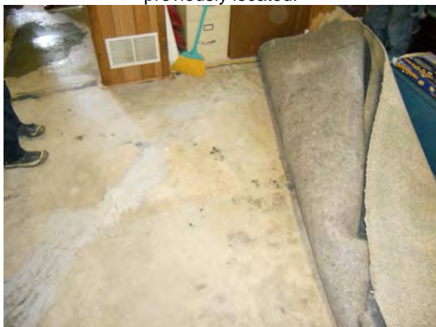
Sealed cracks beneath carpeting in living area.
