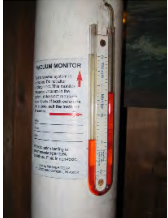
Radon System – Structure 39
