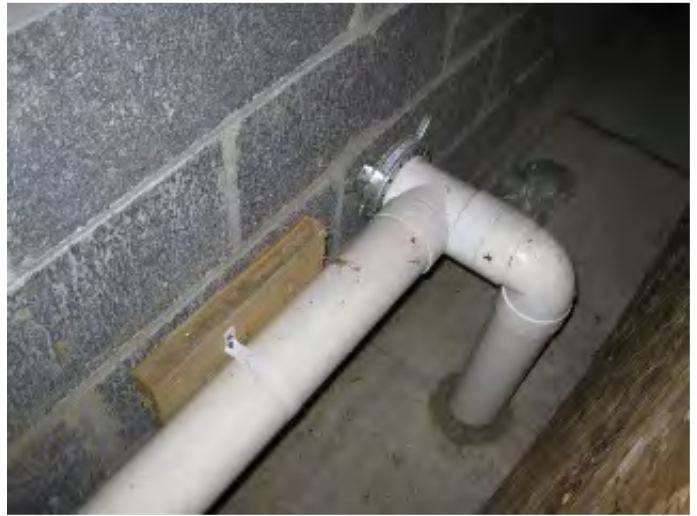
Radon System – Structure 35
