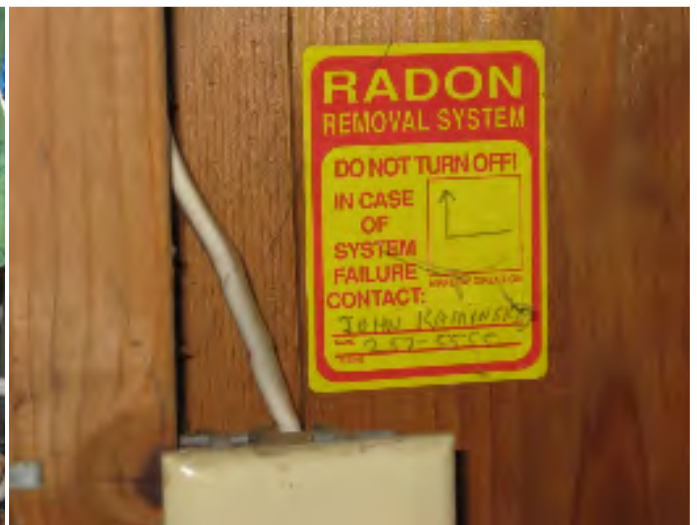
Radon System – Structure 39
