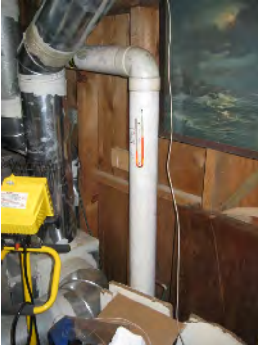
Radon System – Structure 39
