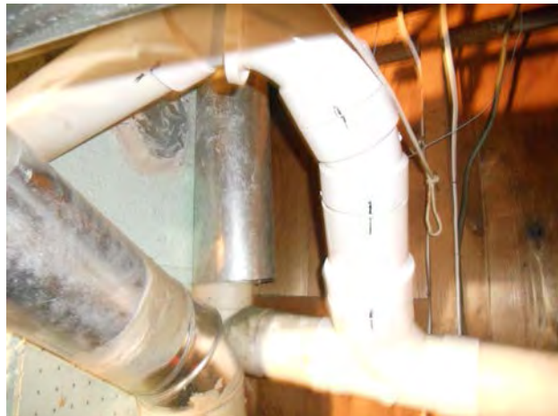
Connection of EP-2 to existing SSDS line in Structure 39
