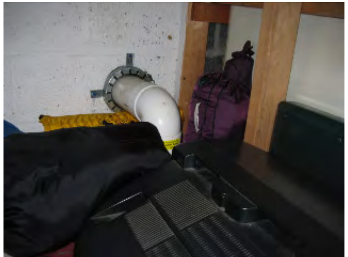
Radon System – Structure 35
