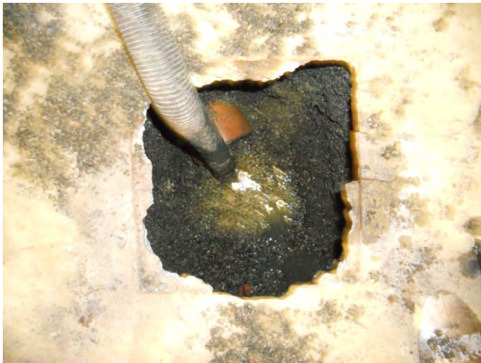
Unsealed, open floor drain – Structure 35
