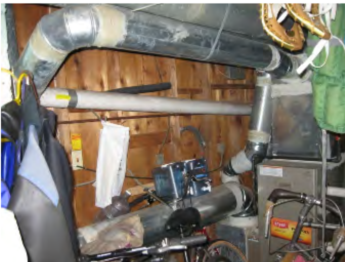
Radon System – Structure 39
