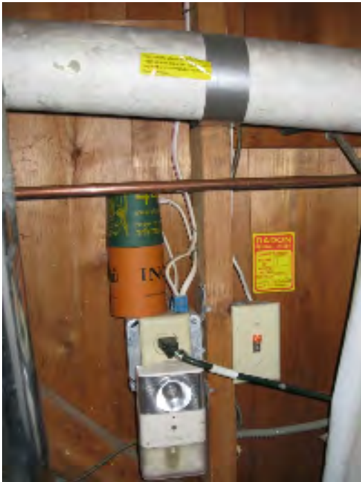
Radon System – Structure 39
