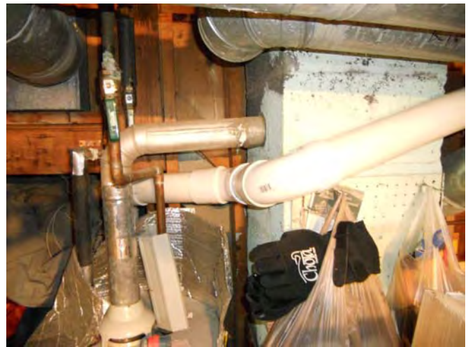
Piping around water heater and chimney to existing line.
