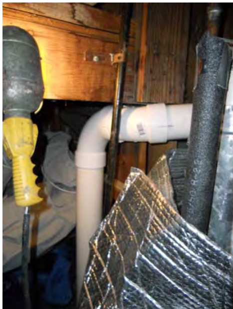
Extraction point and piping around water heater.
