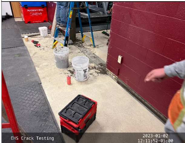
Transition piece, entering Room 143. Crack/opening.
