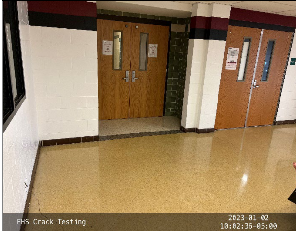
Observed crack, adjacent to Office 141.
