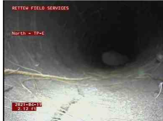
2, 00:00:00, 0.00ft Special Chamber / TP-E
