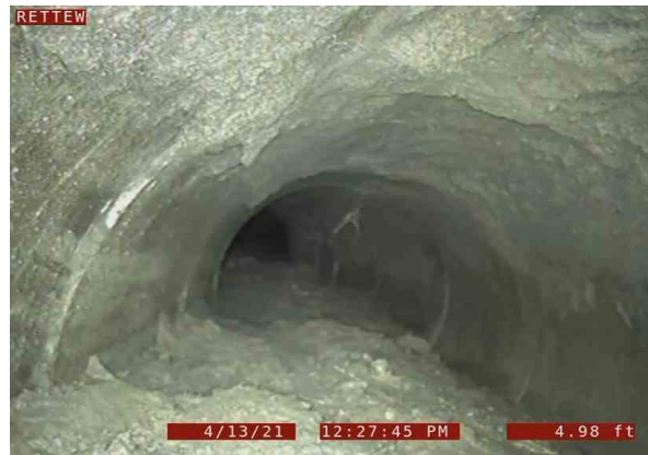
4, 00:12:58, 4.98ft Deposits Settled Fine, 50% of cross sectional area from 3 o'clock to 9 o'clock, Finish
