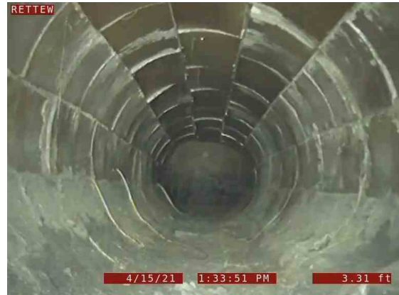
4, 00:01:31, 0.00ft Roots Medium Barrell from 4 o'clock to 10 o'clock, 5% lost, Start
