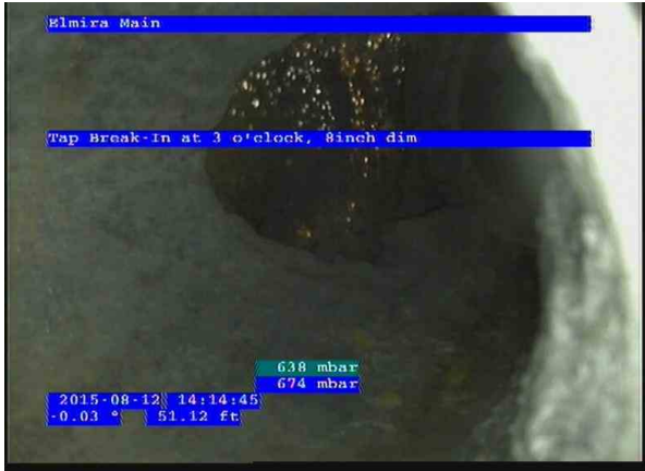
cb1 to tp9_0b14f4d2-d1c7-4454-a854-ed68ed522aaa_20191227_17 2057_095.jpg, 00:02:56, 51.12ft Tap Break-In at 3 o'clock, 8inch dim
