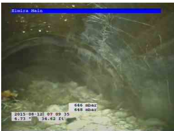
Test Pit 3 to CB24_193ac897-ba82-42a1-8636-2d8ac1facbb_20200116_203846_891.jpg, 00:15:21, 35.00ft Deposits Ingress Gravel, 100% of cross sectional area from 12 o'clock to 12 o'clock, within 8 inch
