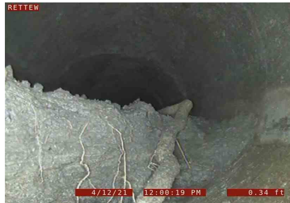
4, 00:00:30, 0.30ft Deposits Ingress Gravel, 40% of cross sectional area from 5 o'clock to 9 o'clock
