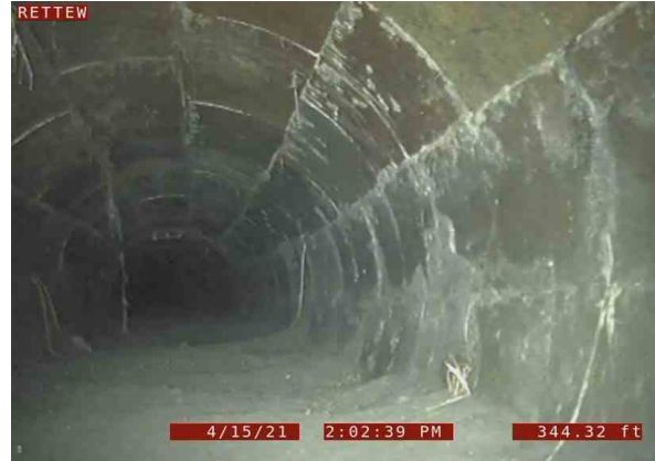
6, 00:09:23, 344.00ft Deposits Settled Fine, 25% of cross sectional area from 4 o'clock to 8 o'clock, Start
