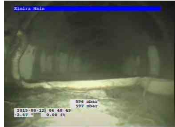
Test Pit 3 to CB24_4385de2d-c372-4285-972d-a1a498ae8a72_20200116_203933_753.jpg, 00:00:08, 30.00ft Roots Tap Barrell from 4 o'clock to 8 o'clock, 10% of cross sectional area, within 8 inch, Finish / Restricted Robot Movement
