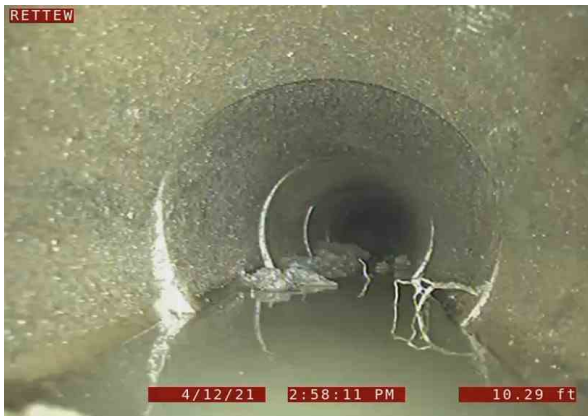
3, 00:00:47, 10.00ft Deposits Ingress Fine, 25% of cross sectional area from 6 o'clock to 9 o'clock, Start
