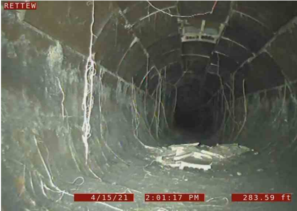
5, 00:08:02, 295.00ft Broken at 12 o'clock
