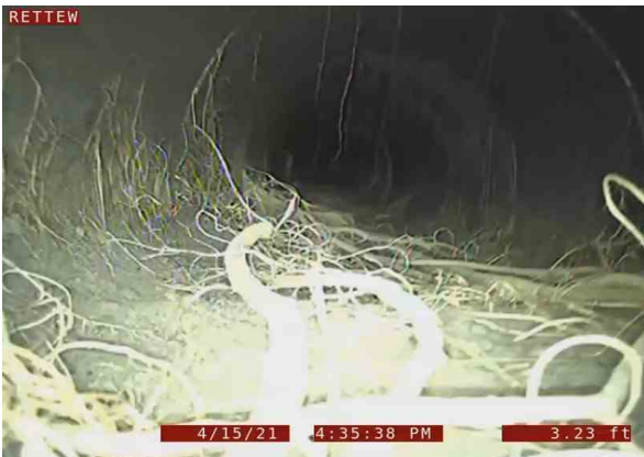
3, 00:00:21, 0.00ft Roots Tap Barrell from 4 o'clock to 8 o'clock, 15% of cross sectional area, Start
