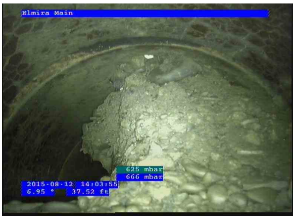
CB1 to North_34b2221a-9bc8-45a6-be9f-adab65d65e17_20191227_171006_857.jpg, 00:01:25, 37.52ft Deposits Ingress Gravel, 85% of cross sectional area from 11 o'clock to 7 o'clock, within 8 inch
