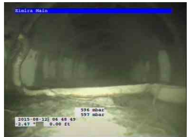
Test Pit 3 to CB24_e0451d6a-9a20-41c9-807d-15aefa77ebb6_20200116_203414_514.jpg, 00:00:08, 0.00ft Roots Tap Barrell from 4 o'clock to 8 o'clock, 10% of cross sectional area, within 8 inch, Start / Restricted Robot Movement
