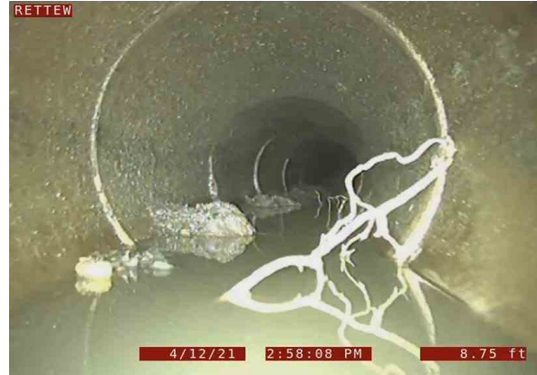
2, 00:00:23, 8.75ft Roots Tap Joint at 3 o'clock, 5% of cross sectional area, within 8 inch
