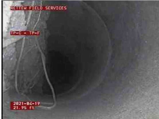
5, 00:05:15, 21.00ft Deposits Settled Fine, 30% of cross sectional area from 3 o'clock to 9 o'clock, Finish
