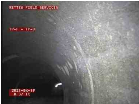
3, 00:00:31, 0.50ft Survey Abandoned / DSF
