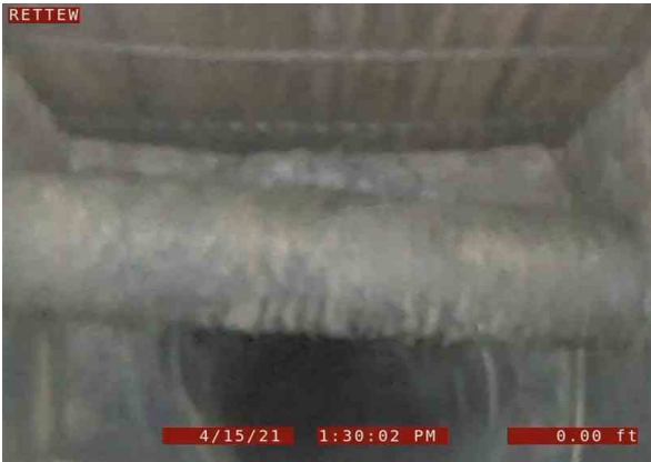
3, 00:00:00, 0.00ft General Observation / Cross Bore in Manhole Chamber
