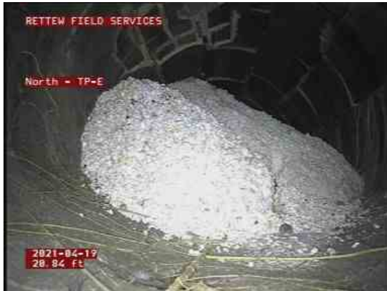
3, 00:00:55, 21.00ft Deposits Settled Fine, 50% of cross sectional area from 3 o'clock to 9 o'clock / Grout, Bentonite Clay
