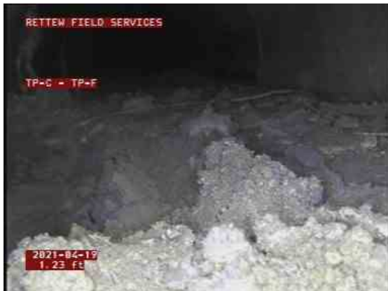
3, 00:00:22, 5.00ft Roots Tap Joint at 9 o'clock, 25% of cross sectional area, within 8 inch
