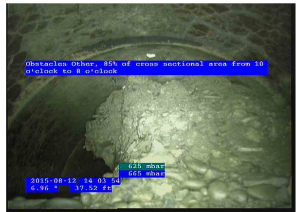
CB1 to North_f745a7d9-1f96-485b-b468-2b0fa75d1210_20191227_171005_621.jpg, 00:01:22, 37.52ft Hole Soil Visible at 12 o'clock, within 8 inch, 3inch defective
