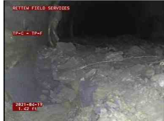
2, 00:00:22, 0.00ft Deposits Settled Fine, 30% of cross sectional area from 3 o'clock to 9 o'clock, Start
