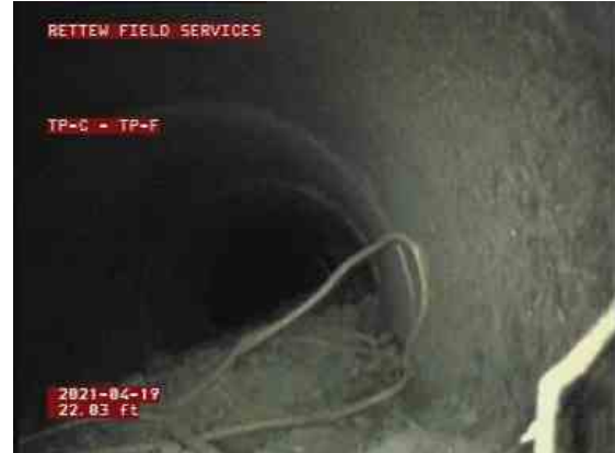
6, 00:05:15, 21.00ft Obstacles Other, 30% of cross sectional area from 4 o'clock to 8 o'clock / DSF
