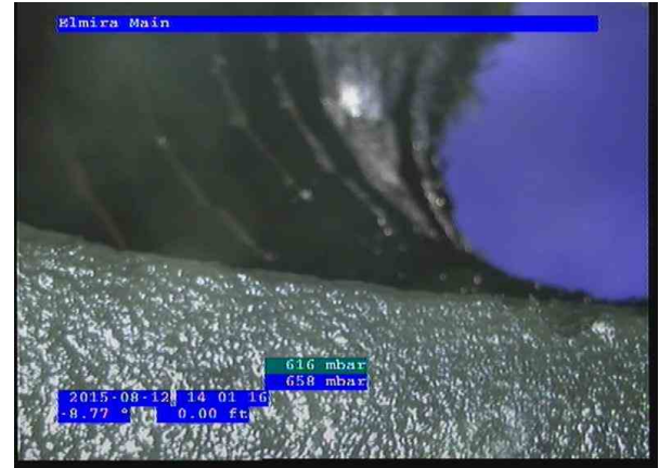
CB1 to North_345adc86-a8bd-4351-ae98-2526a00ef8ff_20191227_170727_418.jpg, 00:10:55, 0.00ft Catch Basin / CB1 Start
