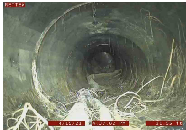
4, 00:01:44, 21.00ft Roots Tap Barrell from 4 o'clock to 8 o'clock, 15% of cross sectional area, Finish
