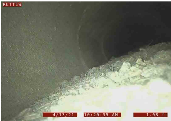
3, 00:00:18, 1.00ft Deposits Settled Fine, 50% of cross sectional area from 3 o'clock to 9 o'clock, within 8 inch, Start
