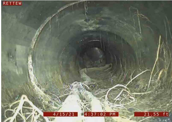
5, 00:01:44, 21.50ft Obstacles Other, 15% of cross sectional area from 4 o'clock to 8 o'clock / RTB
