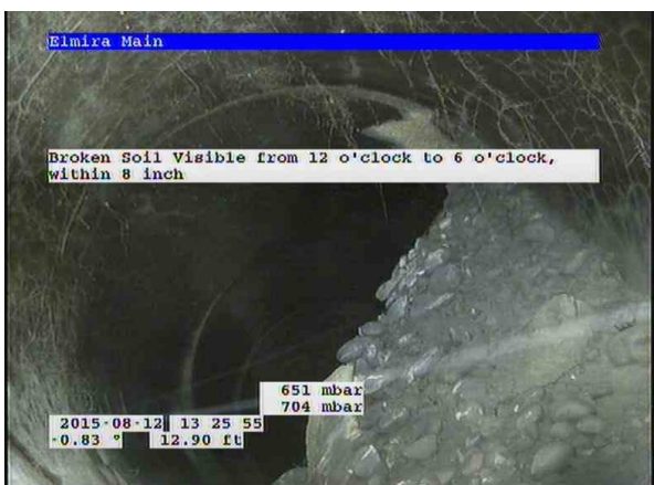
tp7 to cb24_6fc84e18-5cff-42e2-a8e7-d1007cb0572a_20191227_16 2307_412.jpg, 00:03:05, 12.90ft Broken Soil Visible from 12 o'clock to 6 o'clock, within 8 inch
