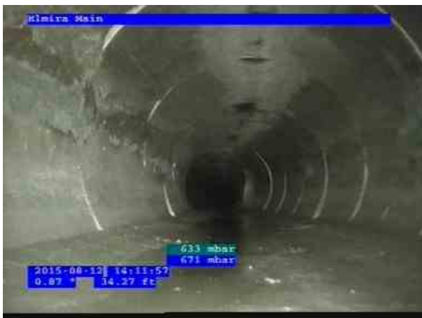
CB-01 to TP-09_e1a0b801-41b1-4691-b8b6-3c378fd5efef_20200116_2 12138_866.jpg, 00:00:36, 0.00ft Deposits Settled Fine, 15% of cross sectional area from 4 o'clock to 8 o'clock, within 8 inch, Start / MUD
