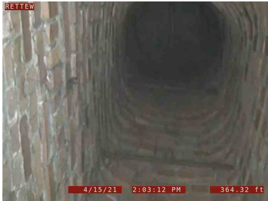
7, 00:00:13, 364.00ft General Observation / MH-40 (Buried)
