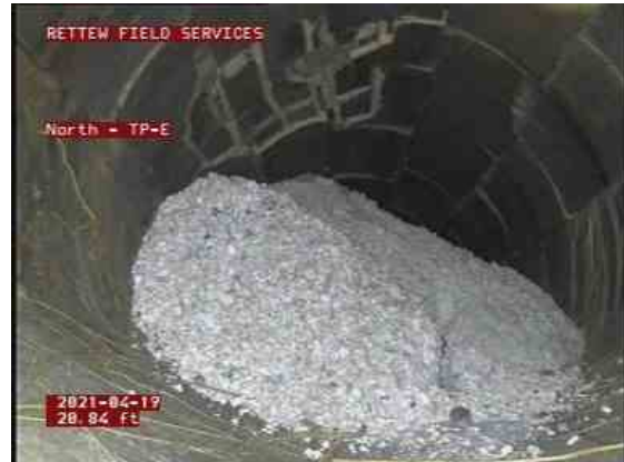
4, 00:00:55, 21.00ft Survey Abandoned / DSF
