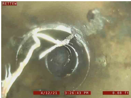
3, 00:00:18, 0.00ft Roots Tap Barrell at 12 o'clock, 10% of cross sectional area
