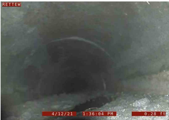
3, 00:00:35, 0.30ft Deposits Ingress Gravel, 50% of cross sectional area from 3 o'clock to 9 o'clock
