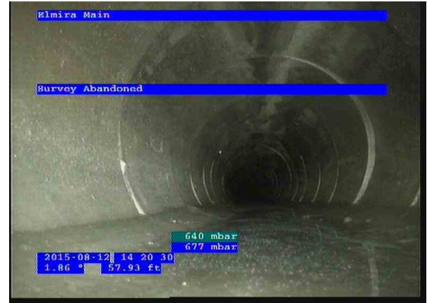
cb1 to tp9_1195476c-1920-4552-8019-c3f8c9076436_20191227_17 2641_971.jpg, 00:07:53, 57.93ft Survey Abandoned / DSF
