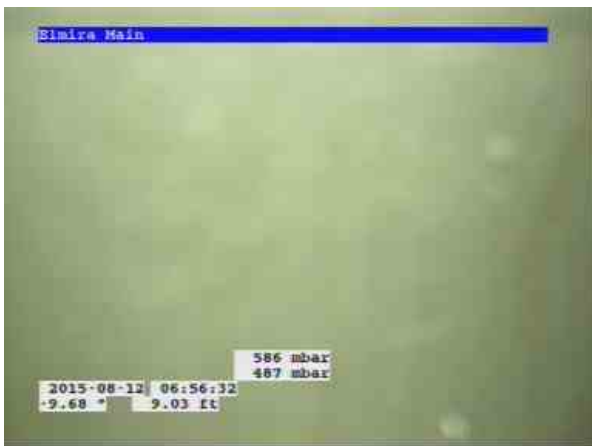
CB-08 to CB-05_7918116b-a89f-4947-a85a-91bfc2f12073_20200116_2 05255_403.jpg, 00:07:22, 9.03ft Tee Connection at 12 o'clock, 12"inch vertical
