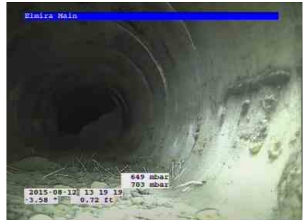
TP-07 to CB-24_272ee1b9-0713-4031-a3c3-a601bffe9576_20200116_211526_222.jpg, 00:00:39, 0.00ft Deposits Settled Gravel, 15% of cross sectional area from 4 o'clock to 8 o'clock, Start
