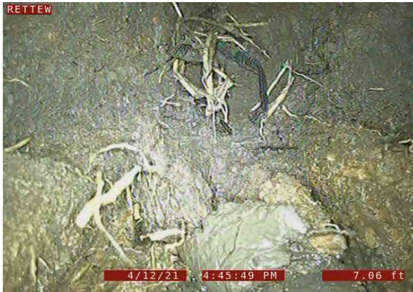
3, 00:00:34, 7.00ft Obstacles Other, 100% of cross sectional area from 12 o'clock to 12 o'clock / Soil and Roots
