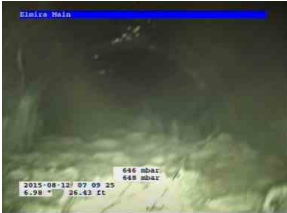
Test Pit 3 to CB24_429c2098-c040-43cc-9dd2-596e8ab088cc_20200116_203628_049.jpg, 00:15:10, 26.00ft Deposits Ingress Gravel, 40% of cross sectional area from 3 o'clock to 9 o'clock, within 8 inch, Start
