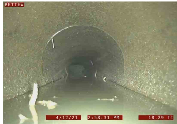
4, 00:00:47, 18.00ft Deposits Ingress Fine, 25% of cross sectional area from 6 o'clock to 9 o'clock, Finish
