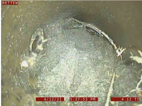
5, 00:03:32, 4.12ft Roots Medium Barrell from 12 o'clock to 12 o'clock, 20% lost
