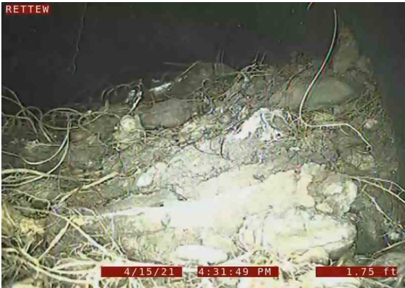
3, 00:00:26, 1.81ft Deposits Ingress Gravel, 80% of cross sectional area from 12 o'clock to 12 o'clock
