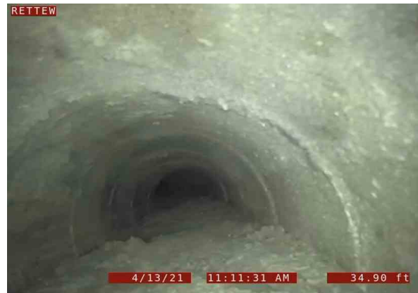
4, 00:00:18, 34.00ft Deposits Settled Fine, 50% of cross sectional area from 3 o'clock to 9 o'clock, within 8 inch, Finish
