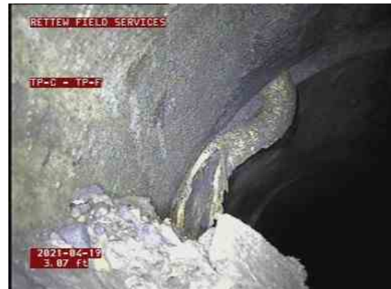
4, 00:00:22, 5.00ft Roots Tap Joint at 9 o'clock, 25% of cross sectional area, within 8 inch
