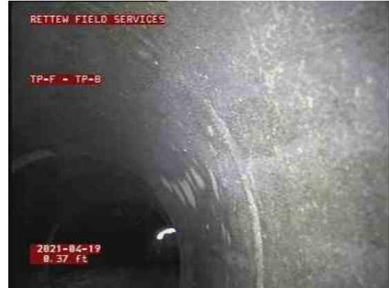
2, 00:00:31, 0.50ft Deposits Settled Fine, 40% of cross sectional area from 4 o'clock to 8 o'clock
