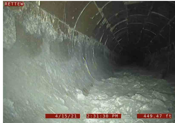
8, 00:01:06, 449.47ft Survey Abandoned / DSF
