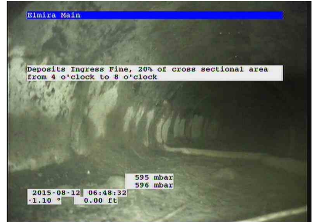
100 ft N CB24_fd7bd9d1-089b-447f-b169-1101e55f2961_20191223_125549_819.jpg, 00:00:00, 0.00ft Deposits Ingress Fine, 20% of cross sectional area from 4 o'clock to 8 o'clock
