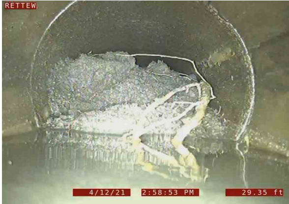
5, 00:01:08, 30.00ft Deposits Ingress Fine, 90% of cross sectional area from 12 o'clock to 12 o'clock
