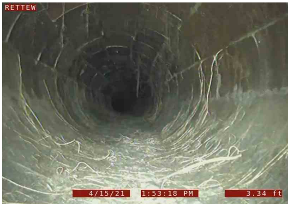
3, 00:00:13, 0.00ft Roots Medium Barrell from 3 o'clock to 9 o'clock, 5% lost, Start
