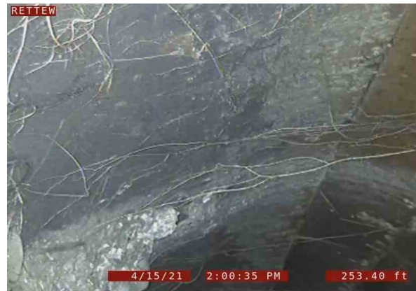
4, 00:07:21, 253.00ft Hole at 10 o'clock
