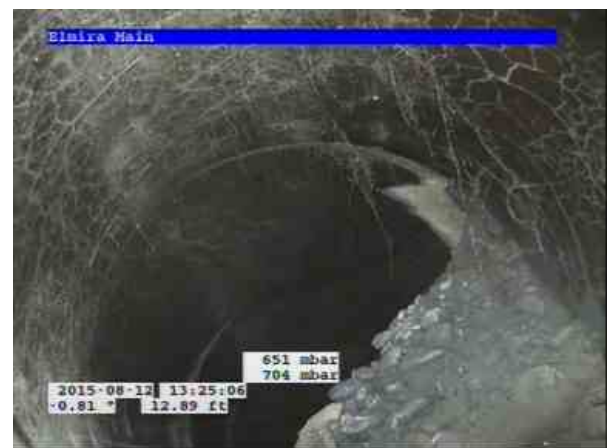
TP-07 to CB-24_6736e719-2d5b-4ac1-88c1-db9eb574c72d_20200116_211026_467.jpg, 00:02:50, 13.00ft Deposits Ingress Gravel, 65% of cross sectional area from 1 o'clock to 7 o'clock, within 8 inch
