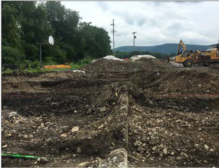
Gas line running through concrete structure
