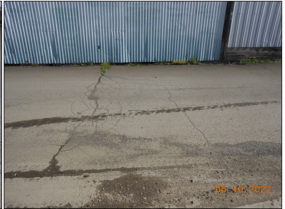
22.) PAOC 17 Bituminous Concrete Crack
