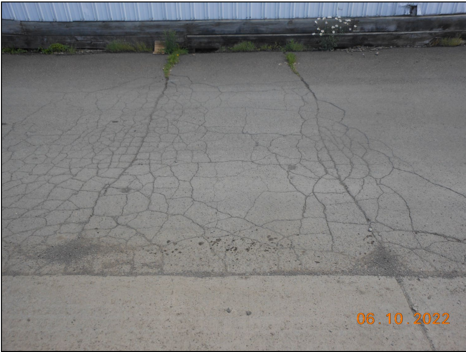
21.) PAOC 17 Bituminous Concrete Cracks
