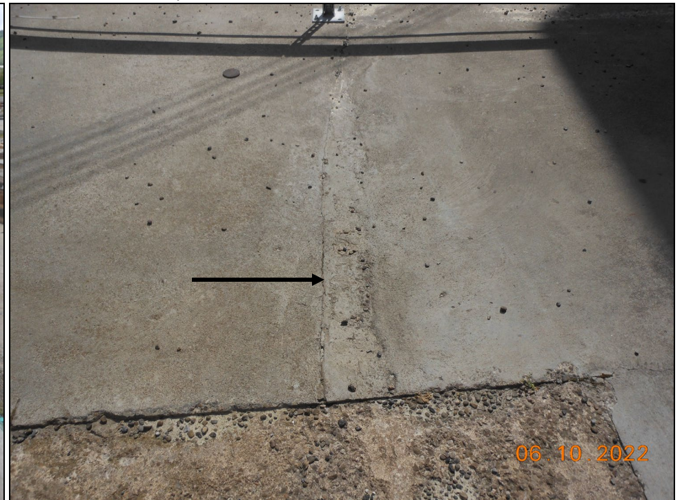
8.) PAOC 8 Concrete Slab Minor Hairline Crack
