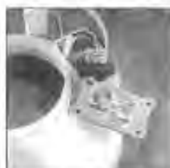
Romex wiring - Top View
