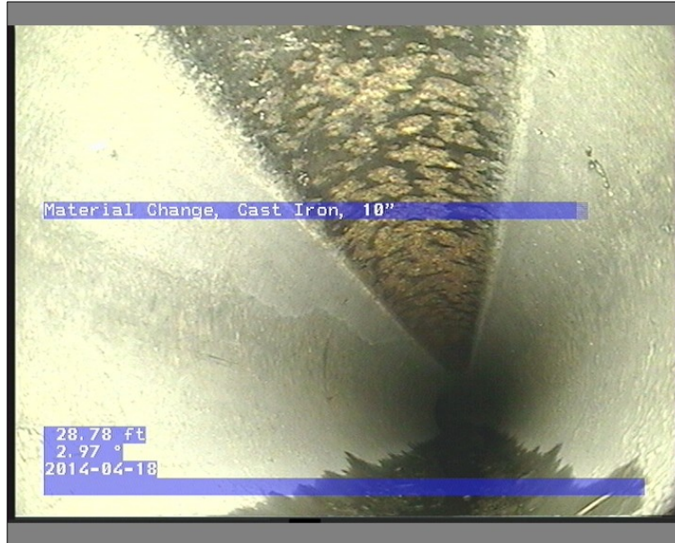
Photo: 4_1_2_18042014_102717_A.JPG, VCR No.: X 30.57FT, Material Change, Cast Iron / 10"
