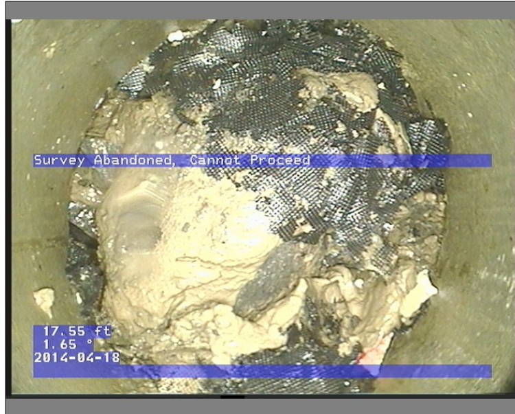
Photo: 5_1_2_18042014_110236_A.JPG, VCR No.: X 17.92FT, Survey Abandoned / Cannot Proceed
