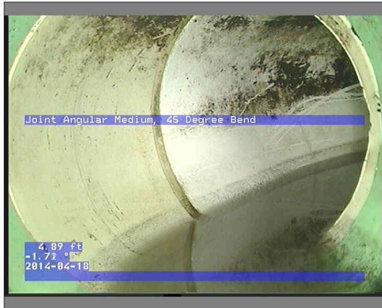
Photo: 6_1_2_18042014_112244_A.JPG, VCR No.: X 4.89FT, Joint Angular Medium / 45 Degree Bend
