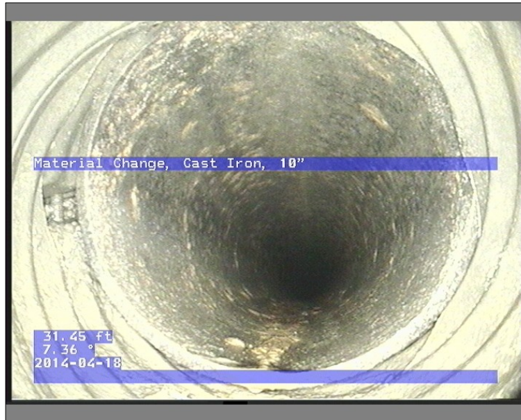
Photo: 2_1_2_18042014_092632_A.JPG, VCR No.: X 34.8FT, Material Change, Cast Iron / 10"
