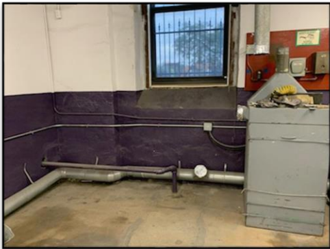
Old water service line (July 1, 2020)
