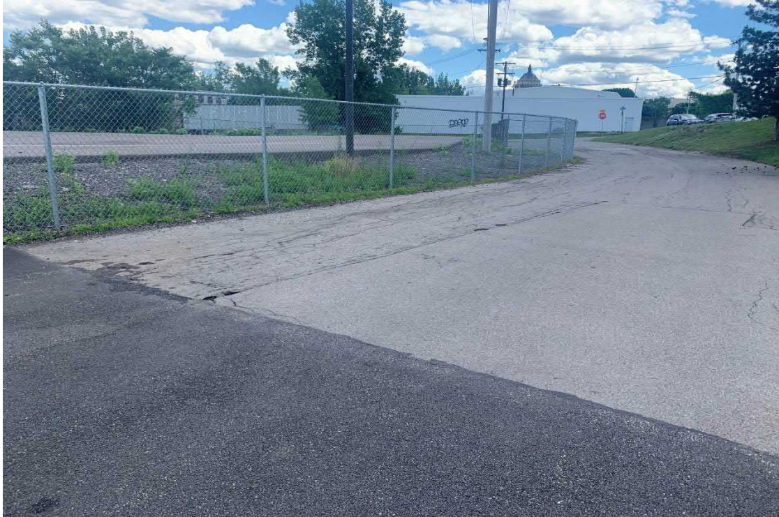
Type 2 Cover Haidt Place and Haidt Place ROW showing cracks.
