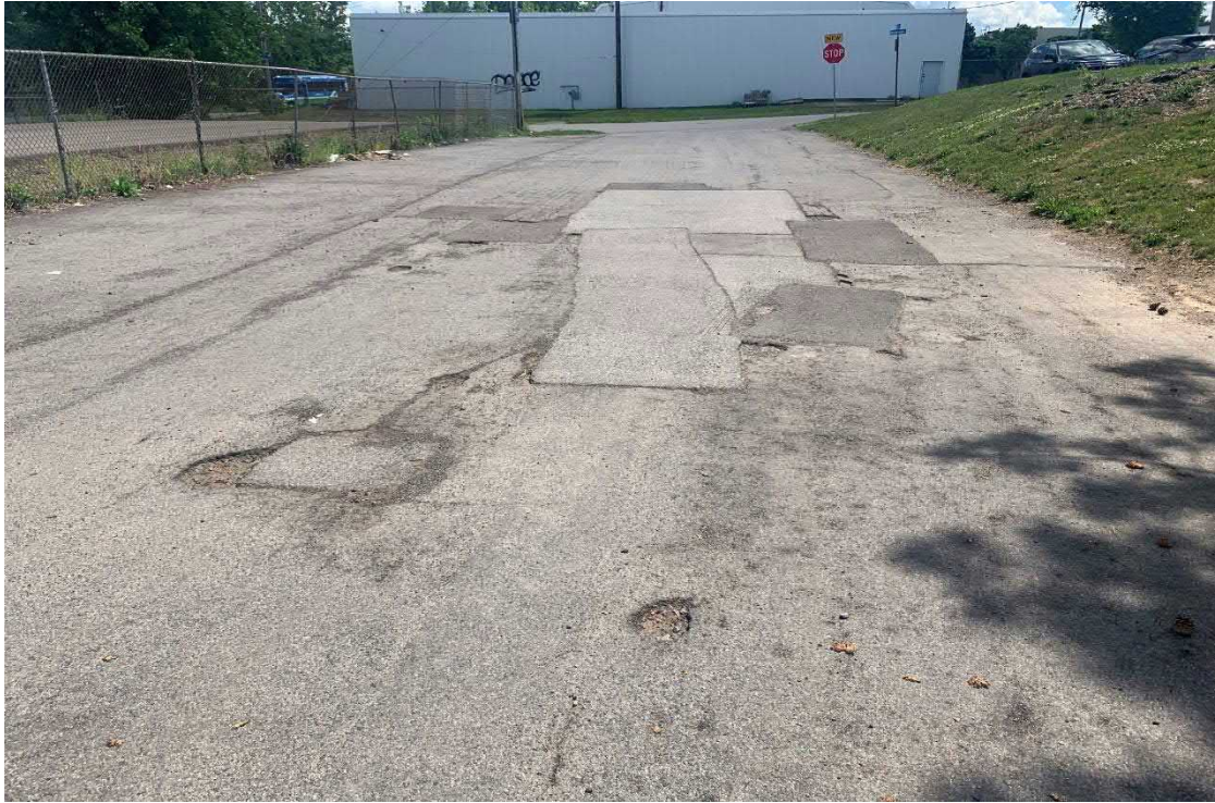
Type 2 Cover with patched area from 2019 and new potholes.
