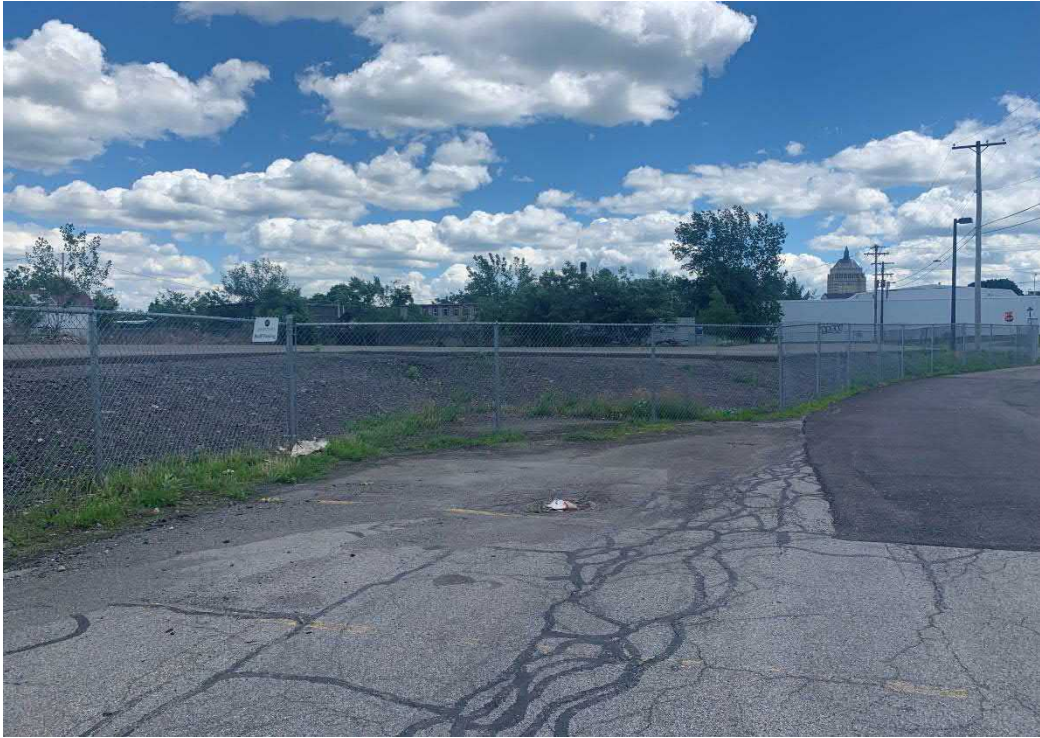
Cover Type 2, view looking south. Debris to be cleared from drain.
