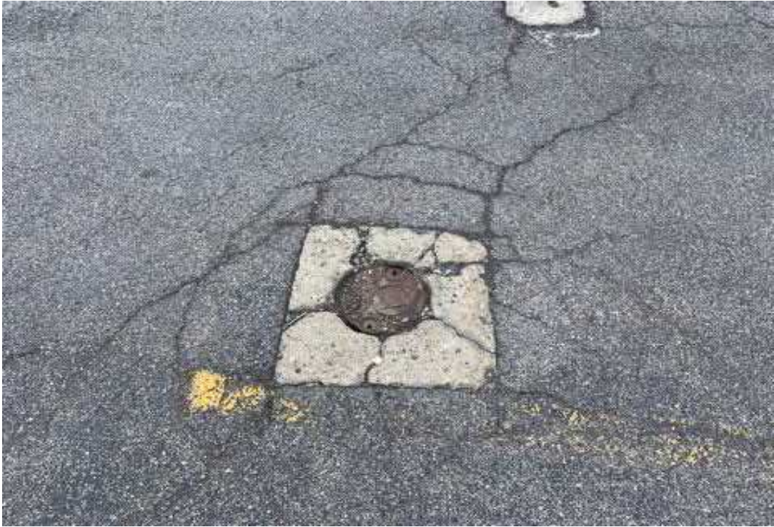
Cracked surface seal/damaged well box at monitoring well MW-101.
