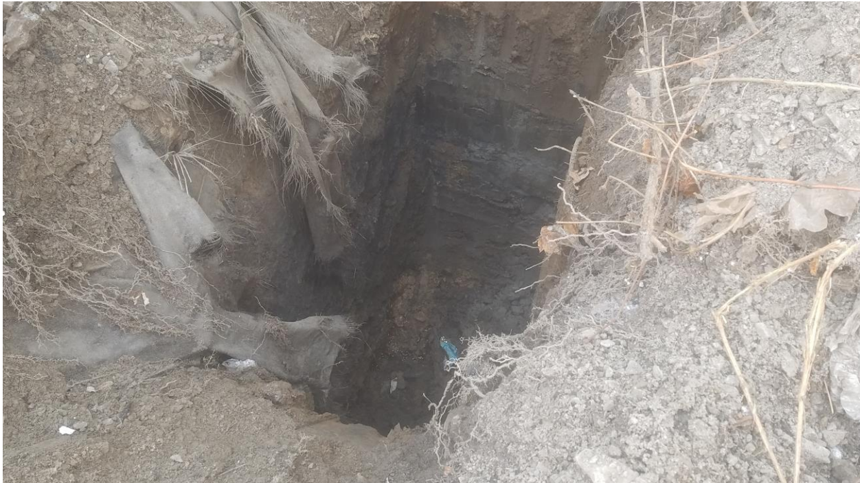
Stained soils in recover well pit
