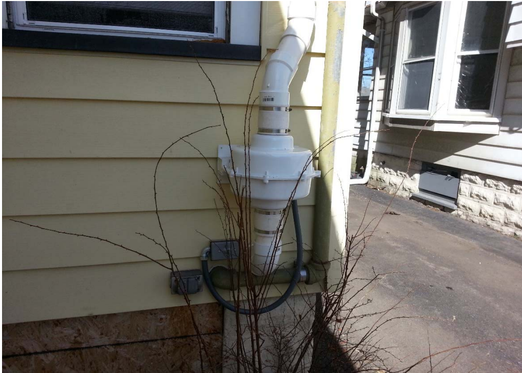
Typical SSD system fan
