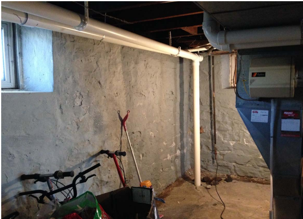
Typical interior SSD system vent pipe and suction point
