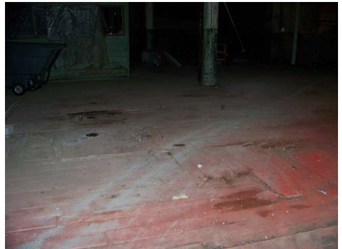
View of the interior wooden floor area with some staining.
