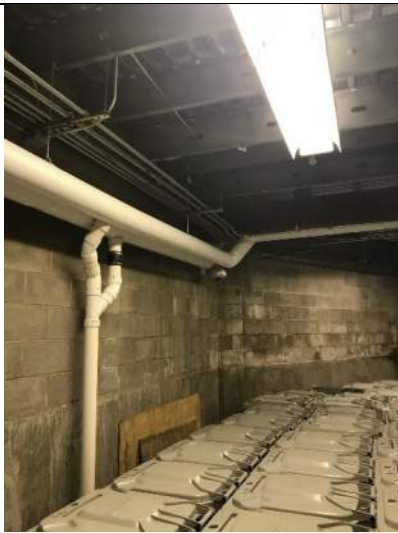
SSDS pipe in loading dock with insulation
