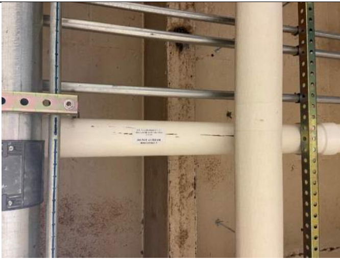
SSDS piping label
