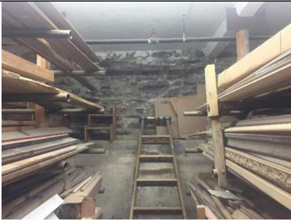
Woodshop basement wall before drylock
