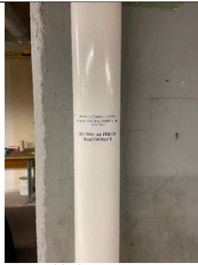
SSDS piping label
