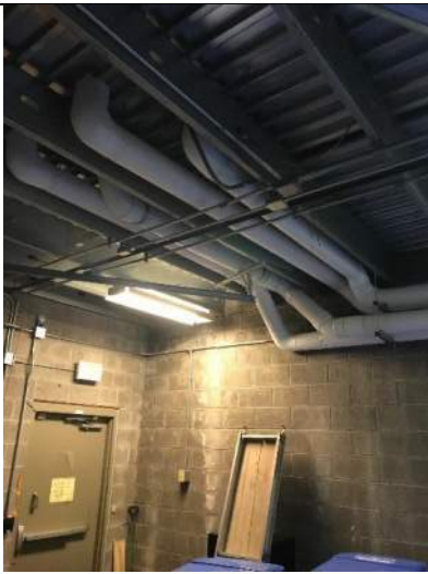
SSDS piping penetrating through loading dock roof to fans
