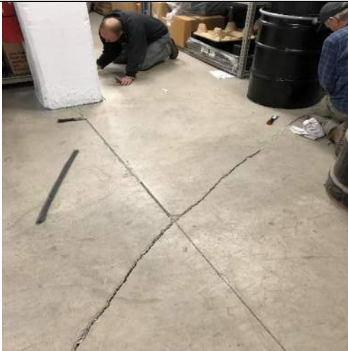
Sealing of crack within floor
