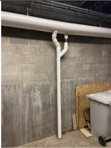
Condensate Drain Pipe in Loading Dock Building
