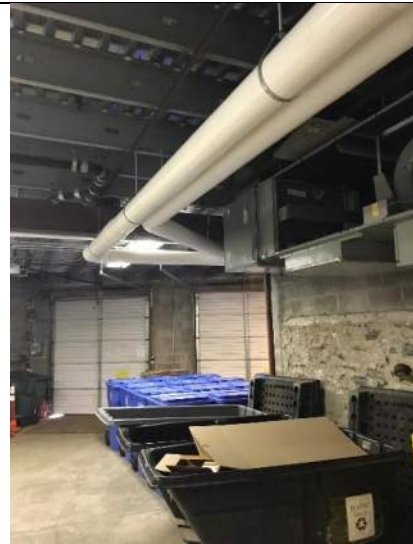
SSDS pipe in loading dock space
