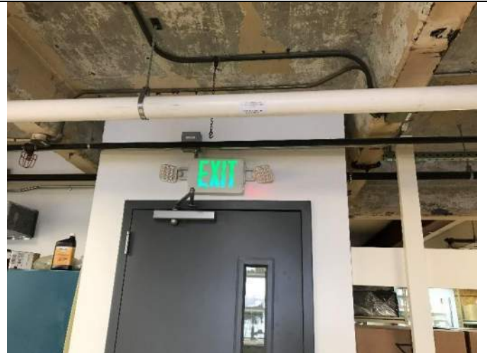
SSDS Lateral and Label identifying pipe
