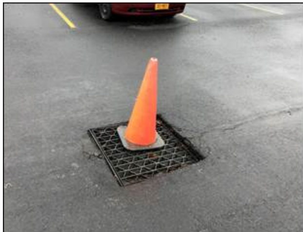
Catch basin in parking lot.
