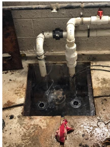
Photo of the sealed, clear polycarbonate cover with two new check valves for drainage into the sump installed in April 2021.
