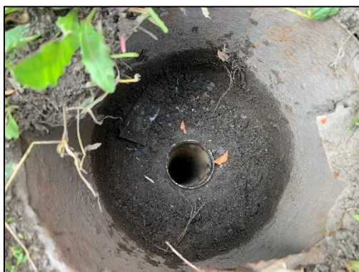
Photo looking down at the warped outer casing and intact inner casing of RW-5 prior to curb box replacement.
