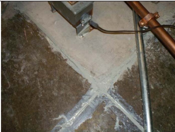
After sealing, saw cuts in the concrete floor slab below the raised floor in the VoltDelta server space.
