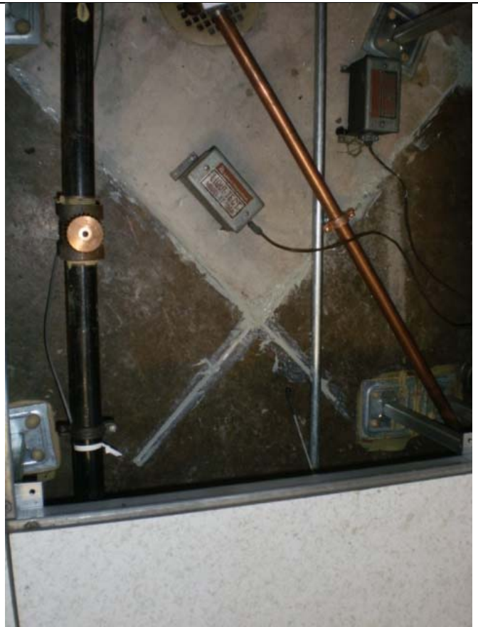
After sealing, saw cuts in the concrete floor slab below the raised floor in the VoltDelta server space.
