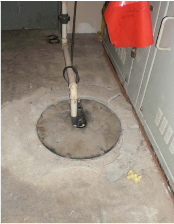
Sump in electrical room, prior to sealing, as found on May 13, 2015 with non-airtight cover.
