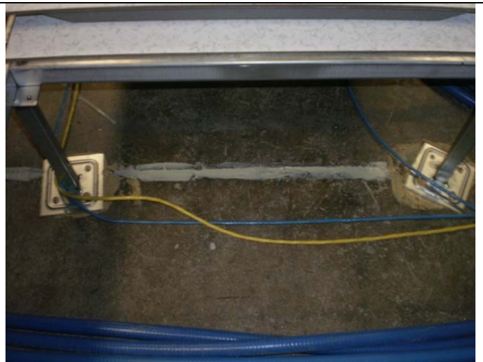
After sealing, an expansion joint in the concrete floor slab below the raised floor in the VoltDelta server space.
