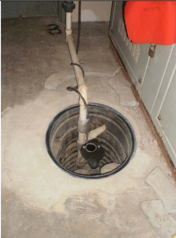
Sump in electrical room after it was sealed with plastic sheeting and check valve assembly on May 13, 2015.
