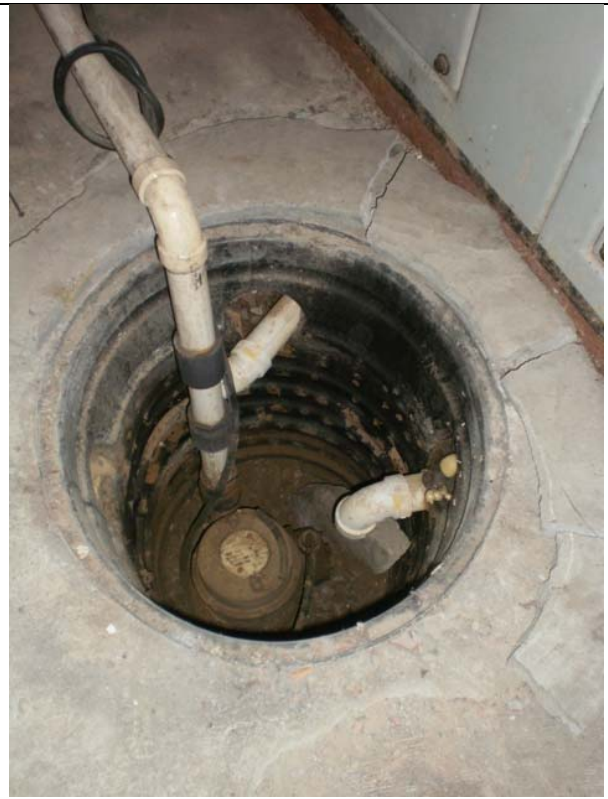
Interior of sump in electrical room, prior to sealing, with non-airtight cover removed.
