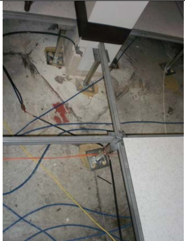
Prior to sealing, typical expansion joints in the concrete floor slab below the raised floor in the VoltDelta server space.
