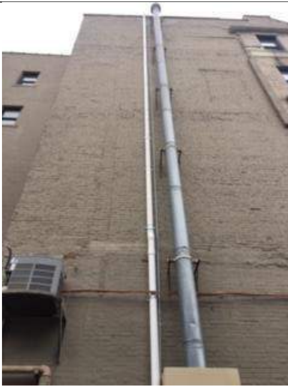
Exterior riser (PVC).
