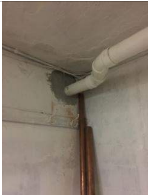
DP-03 - Horizontal depressurization point extending below the western portion of the Site building where no basement is present.
