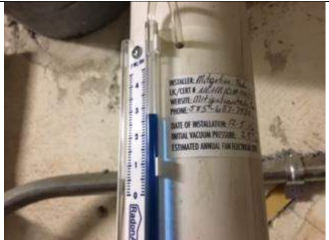
U-tube manometer and label on one of the depressurization points
