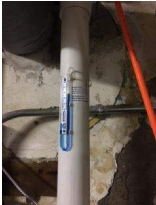
U-tube manometer on one of the depressurization points.
