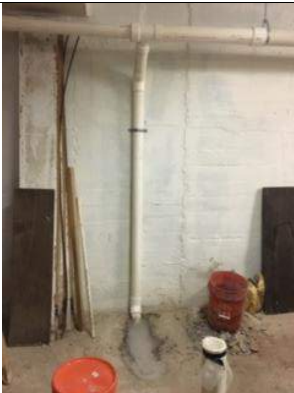
DP-02 - Vertical depressurization point.
