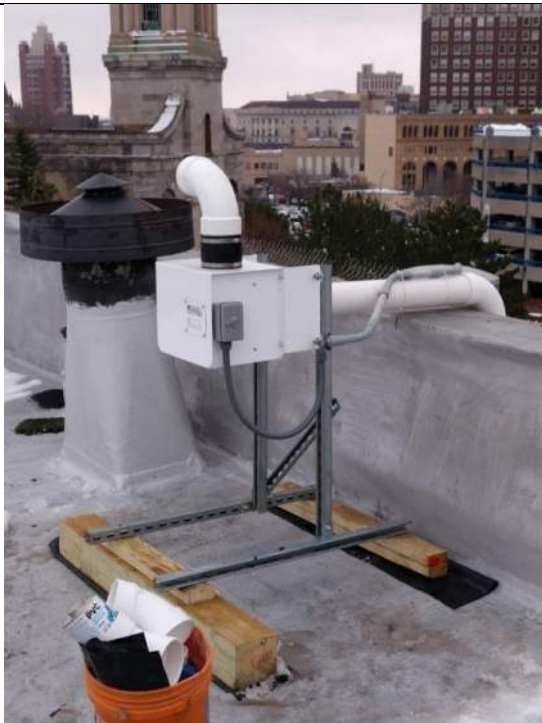
Festa Radon Technologies Company FRT Force fan, located on the roof of the Site building.
