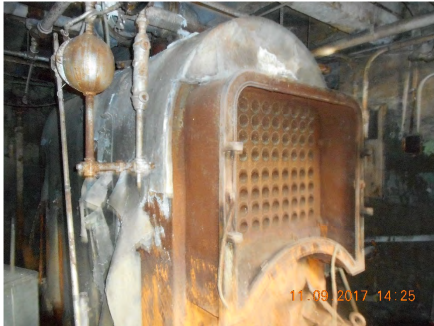
Interior – Basement Boiler
