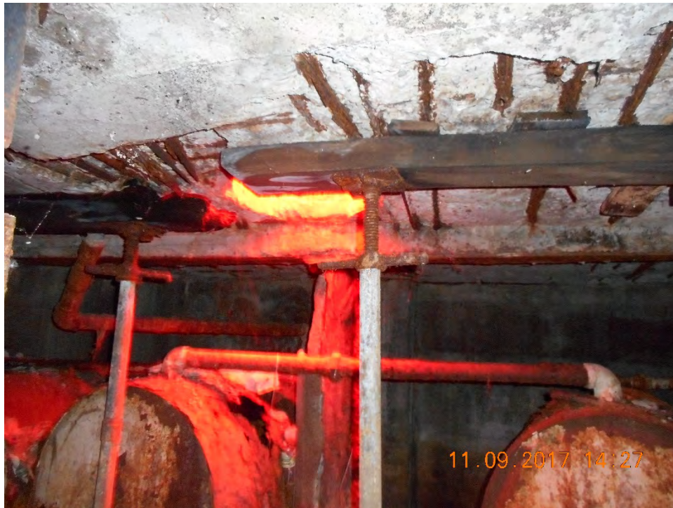
Interior – Basement Vault with ASTs
