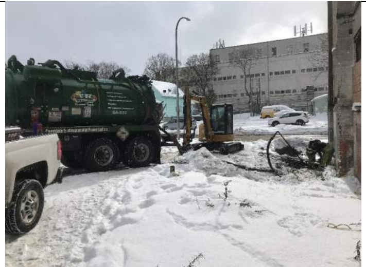
November 13, 2020 – T&R pumping southern UST view looking South.
