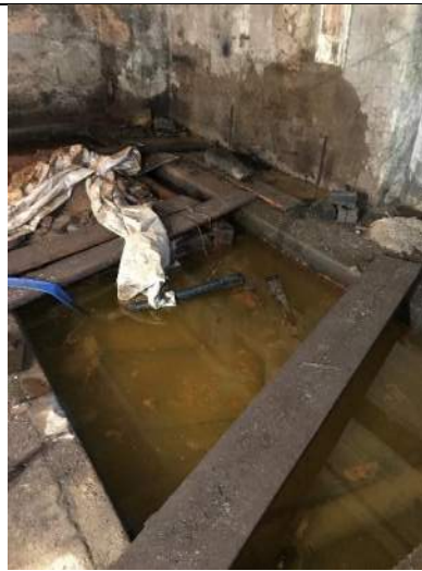
November 25, 2019 – Boiler pit with water and petroleum residue.
