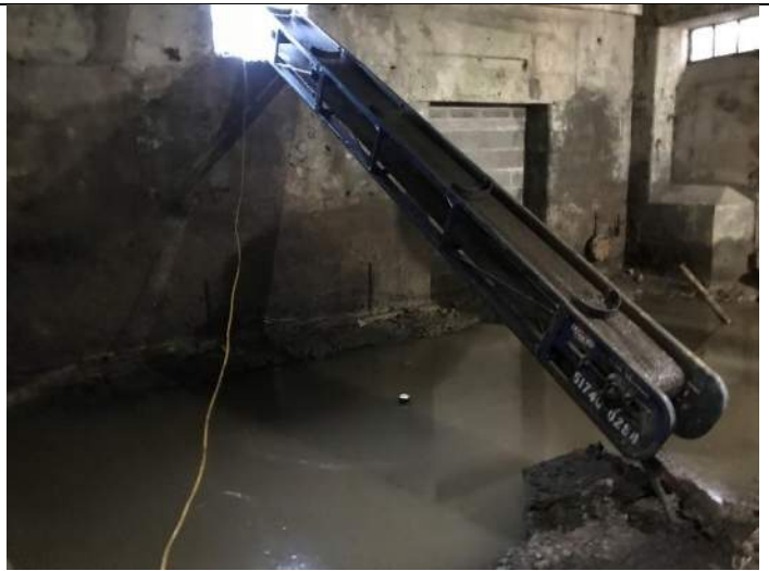
December 30, 2019 – Basement floor removed, water in basement, facing southeast.
