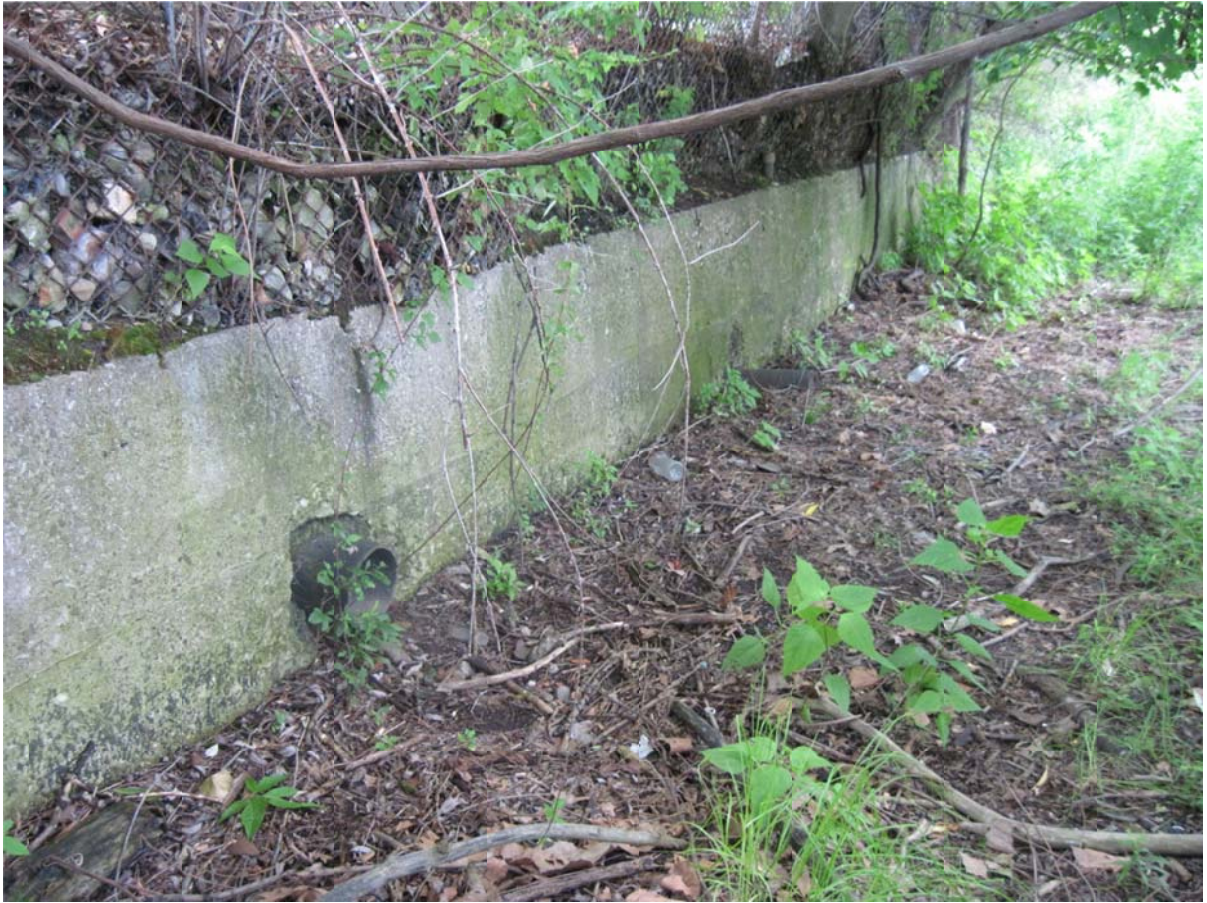
Description: Pipes A and B.
