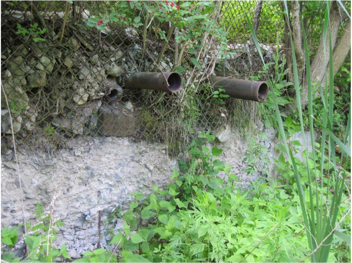
Description: Pipes E.
