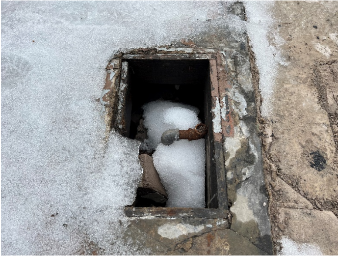
Photo No. 9 Unknown feature connected to subsurface void space
