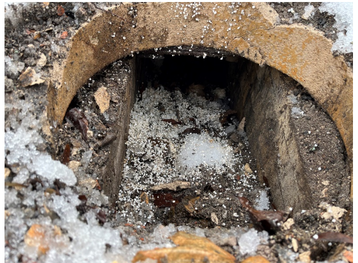
Photo No. 8 Suspect former floor drain inlet
