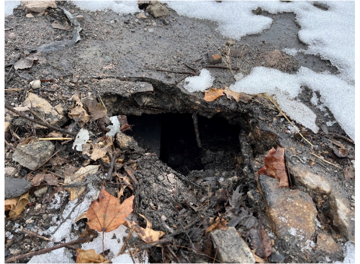
Photo No. 10 Subsurface void space
