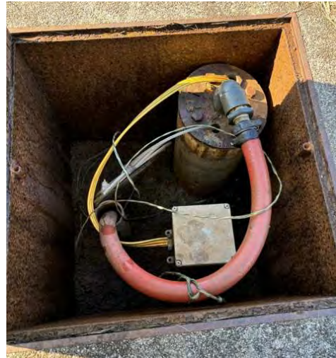
Photo No. 10 Interior of injection well pump.
