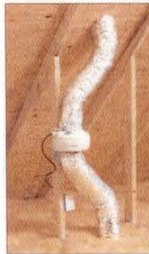
Typical attic installation
