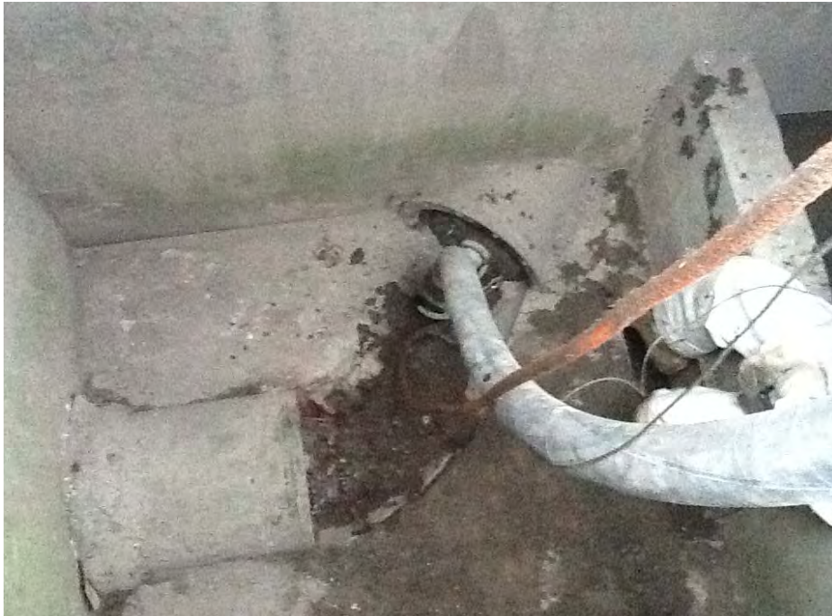
Photograph 5. Filling diversion structure to wet well.
