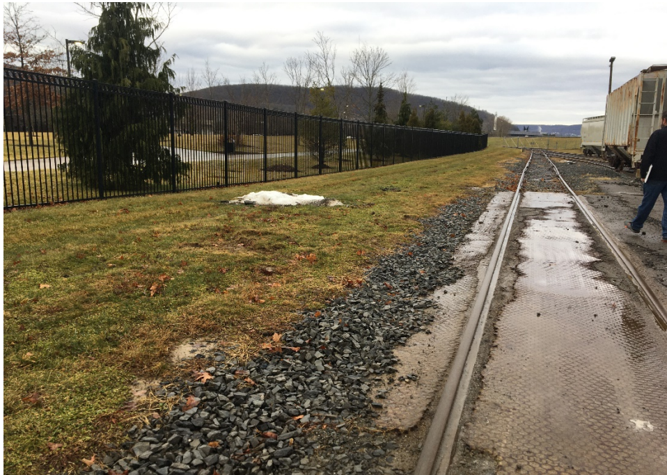
Photo 1: Repaired area of tire rutting in Cover Soil previously noted in 2018 inspection, adjacent to railroad tracks.
