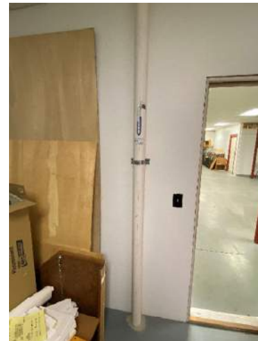
Photo 2: Typical SSDS Suction Pit and Riser
